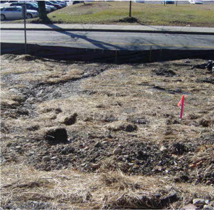
Silt fence was re-installed along Route 1, down gradient from the exposed soil at station #81. The partially mulched soils are susceptible to rill erosion caused by precipitation and surface runoff.
