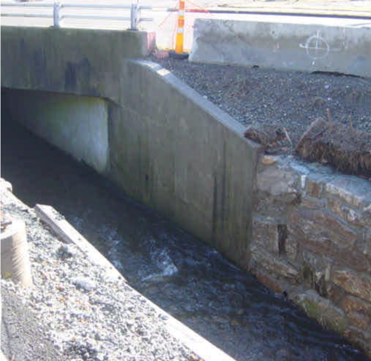
At Stony Brook, the channel remains free of debris. Ensure that soil and gravel at the top of the walls are stable and contained. Work out the final restoration plan.
