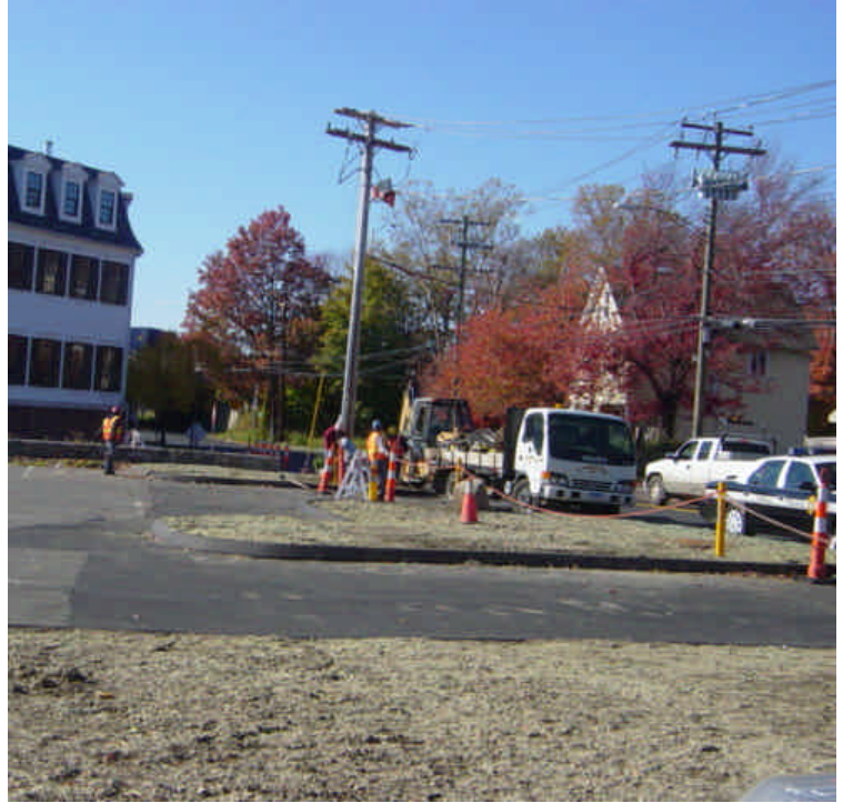
Restoration efforts have been completed near vault #28. The area has been hydroseeded.
