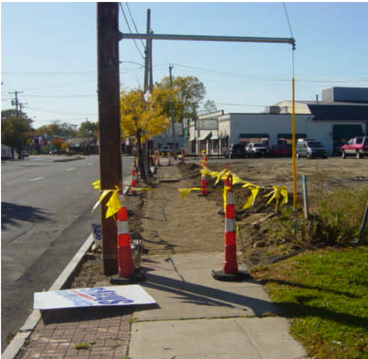
The area near sta. #649 has been prepped for sidewalk restoration. Determine if the vacant lot has been returned to its pre-construction condition. Provide further stabilization if necessary.
