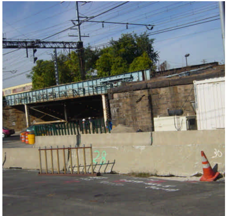
Bridge work, which is not project related, continues near sta. #719. However, the catch basin downgradient should be cleaned as part of the M/N project work.
