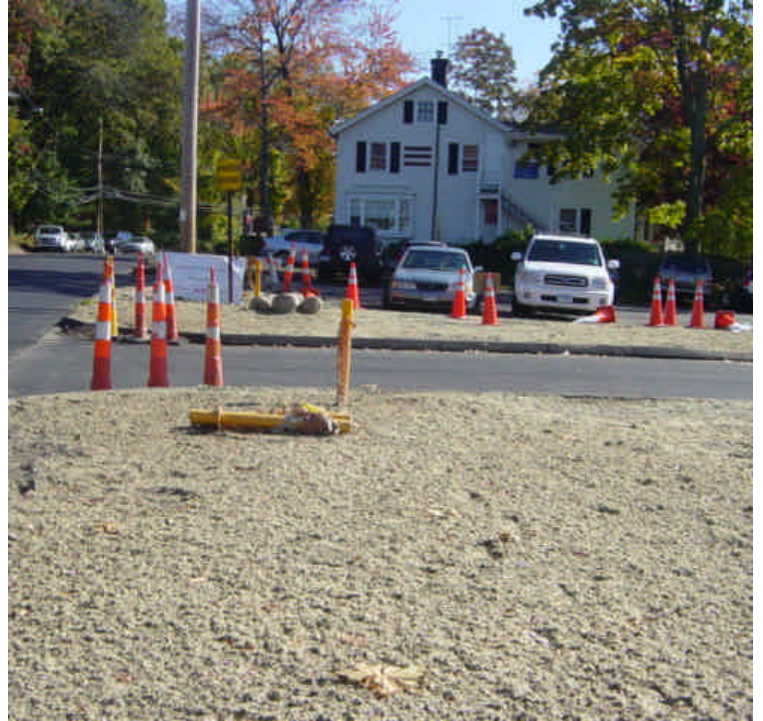
Restoration efforts have been completed near vault #28. The area remains hydroseeded. Monitor for grass cover.
