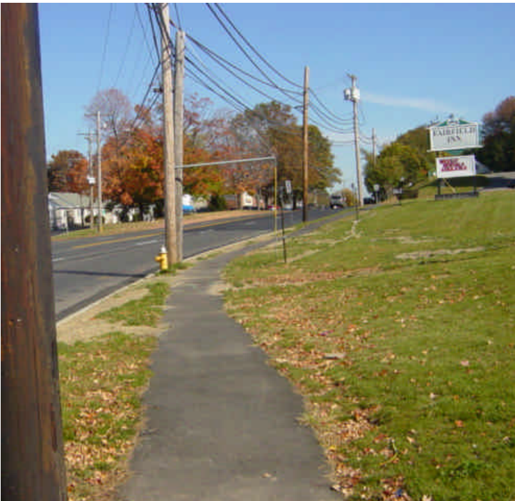
The area near sta. #611 (vault #37) has been partially restored. Small remaining areas of exposed soil have been seeded.
