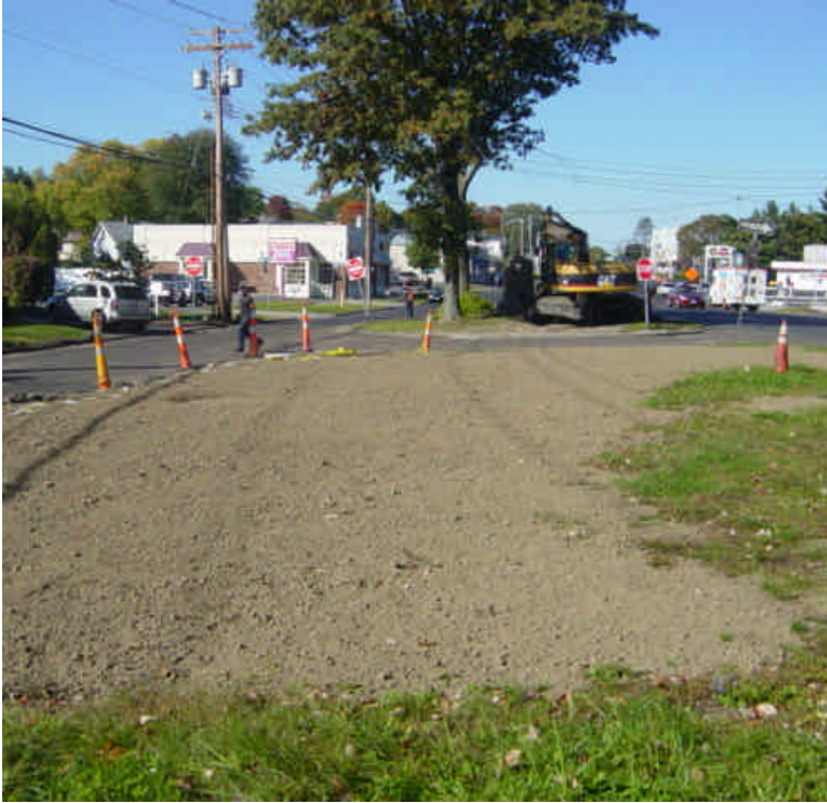
Topsoil has been spread near sta. #463. Ensure the area is properly seeded and mulched to reduce potential for erosion.
