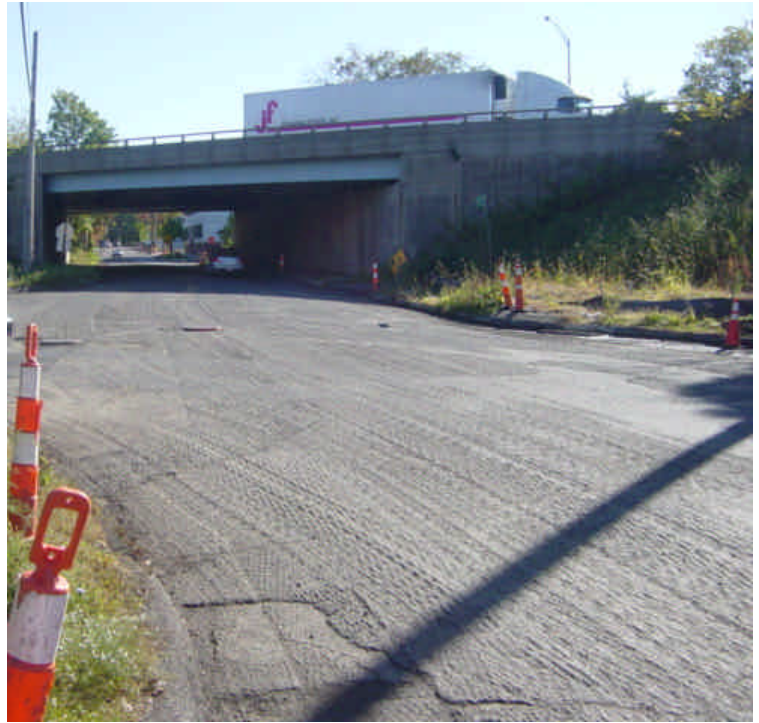
Various portions of Old Post Road have been milled in preparation for final restoration.
