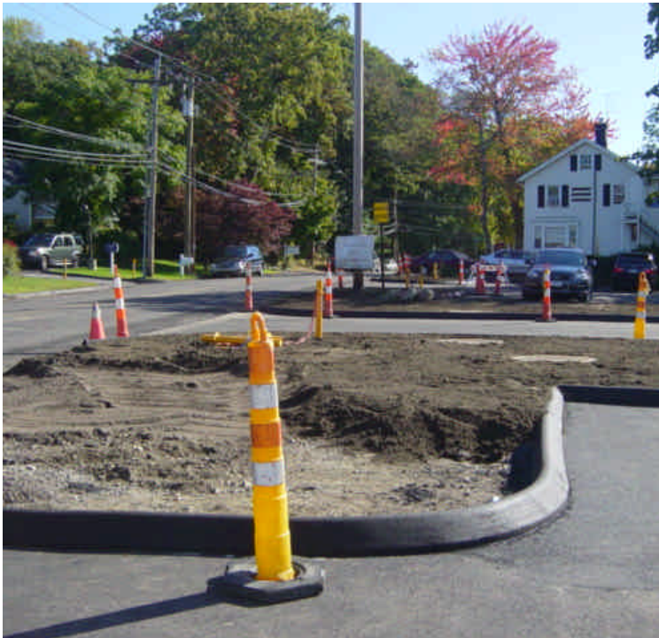
Restoration efforts are underway near vault #28. Ensure topsoil is properly seeded and mulched to reduce potential for erosion.
