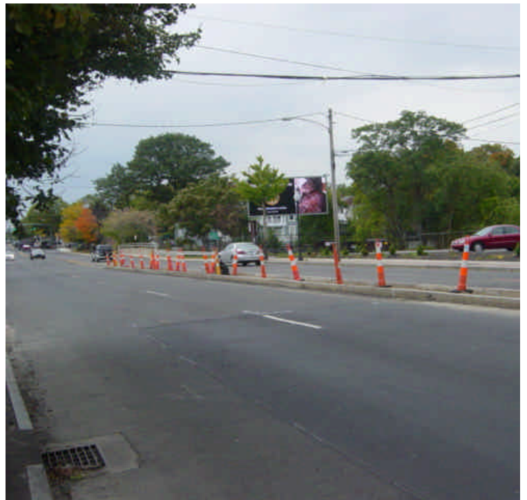
The median was in the process of being restored near sta. #646 along Fairfield Ave.
