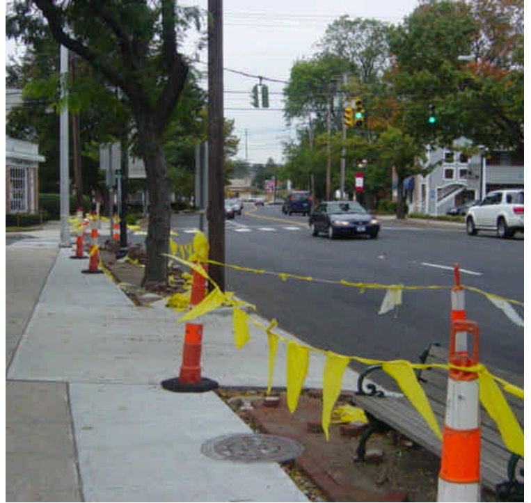
Sidewalk and brick banding pavers have been restored in various locations along Fairfield Ave.
