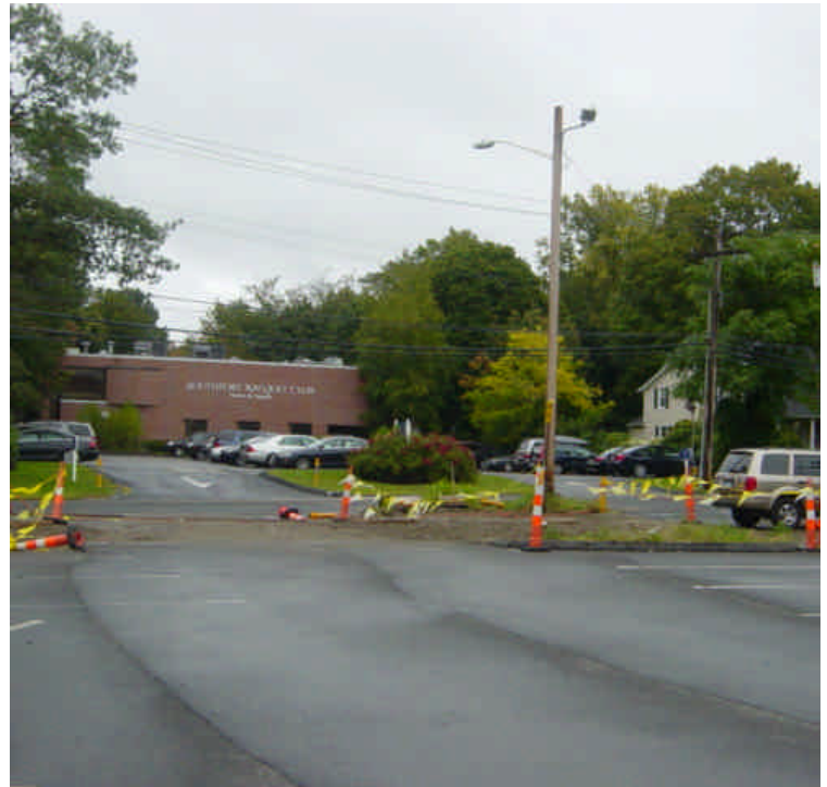
Tie-in work appears to be complete near sta. #28. The area needs to be restored and stabilized.
