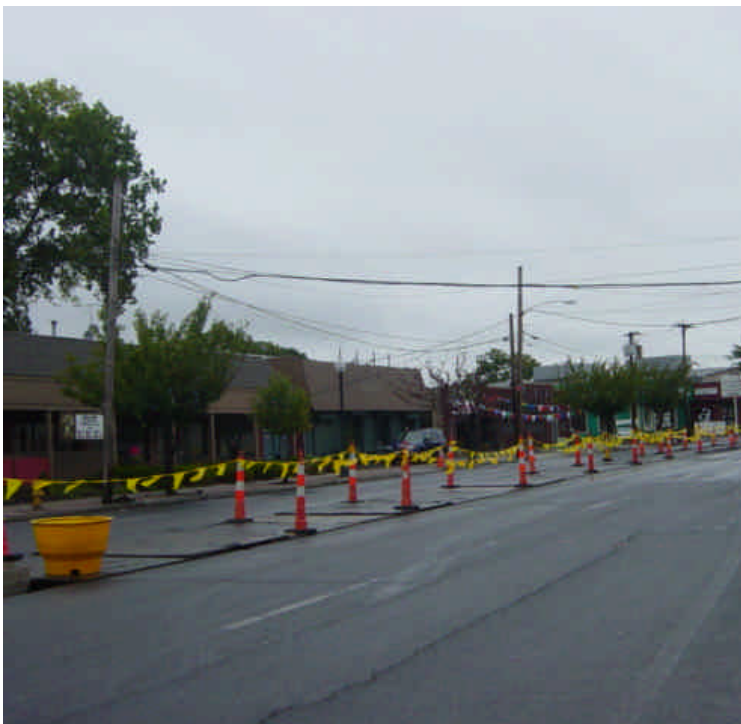
Median and sidewalk restoration was observed in numerous locations along Fairfield Ave.
