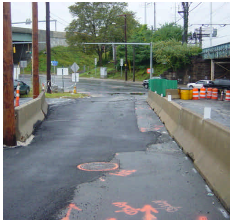
The work area near the intersection of Railroad Ave and Fairfield Ave (sta. #719-720) remains backfilled with process material. Concrete barrier curbs have been placed in the area and the stockpile of sandy material was removed. This work does not appear to be project related. The catch basin should be cleaned.
