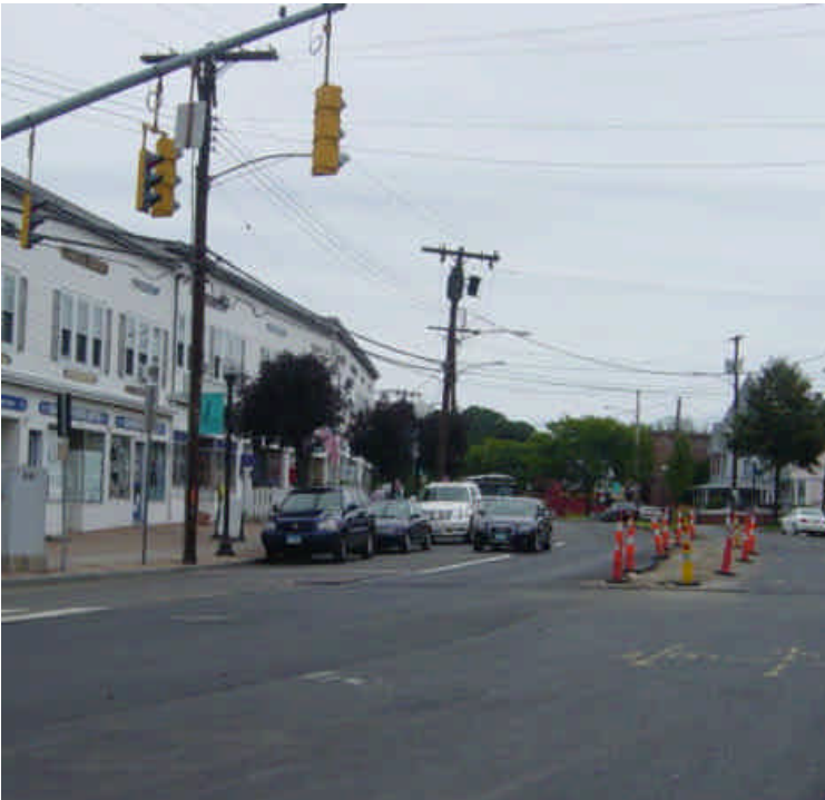
Various portions of Fairfield Ave have been milled in preparation for resurfacing as part of final restoration. Median restoration was also ongoing.
