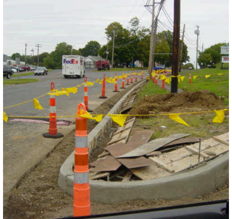
Concrete curbing has been restored near sta. 611 (vault #37). Provide stabilization measures (mulch/stone) to adjacent soil.
