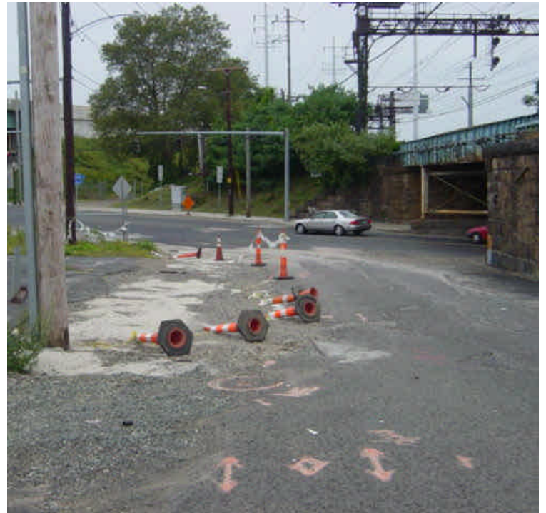
The area near sta. #719-720 remains backfilled with processed material. Some of the material and residual dusty tracking was beginning to be washed onto the roadway and into the catch basin. This may be partially related to utility pole relocation. Sweep, Stabilize, and clean the catch basin.
