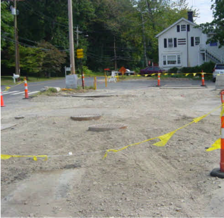
Tie-in work appears to have been completed and vault #28 has been backfilled. The surface remains exposed and should be finalized
