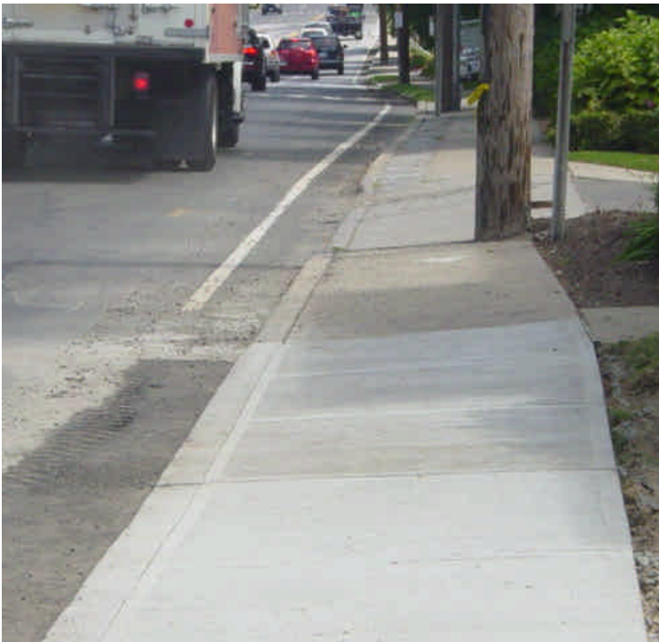
Curbing and sidewalk has been restored near vault #30. A minor amount of cold mix and granular material was observed along the edge of the roadway.
