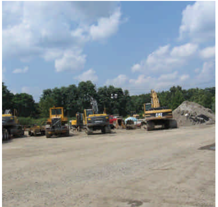
Crushed stone remains throughout the Kings Highway yard to reduce tracking. Sediment tracking and dust migration issues were not observed at the time of the inspection.
