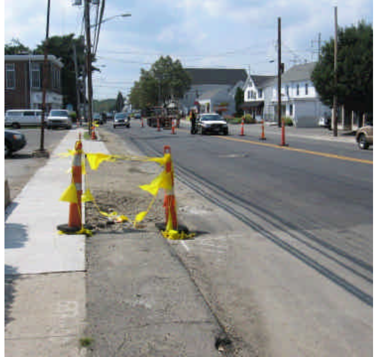
Sidewalk restoration work was ongoing at sta. #535-537. Areas of exposed soil were not contained. Soil has accumulated along the edge of the roadway and needs to be swept.
