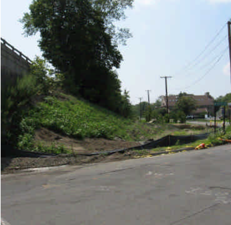
Exposed soil remains along the base of slope near the bridge abutment at sta. #465. Silt fence is falling into disrepair. Provide final stabilization .
