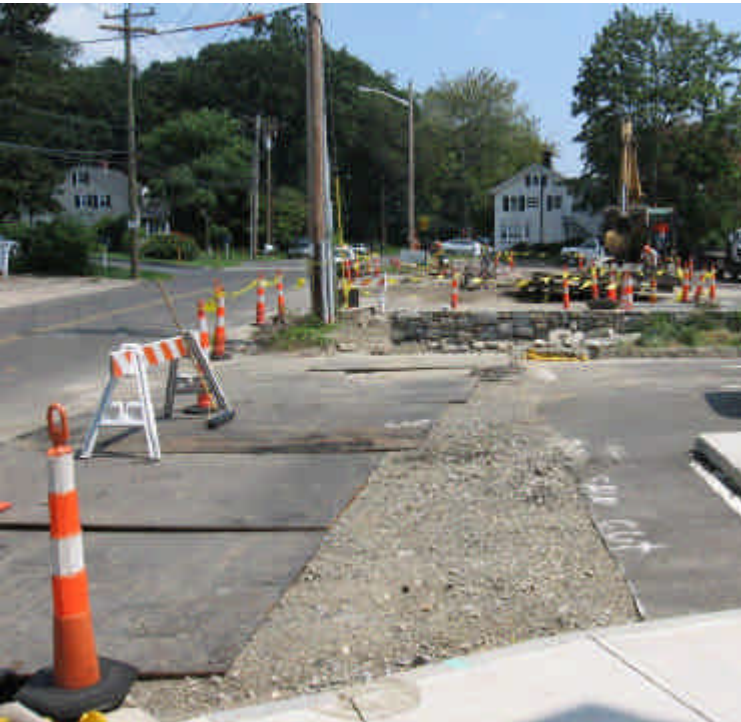
Trenching and tie-in work continues at vault #28. Sweep the Roadway as necessary to prevent tracking.
