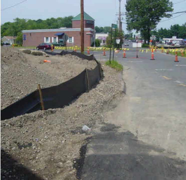
Trenching work is complete near sta. #465. Silt fence has been installed along the curbline. Soil has been stockpiled against the fabric which is stressing it and causing it to rip in some areas.
