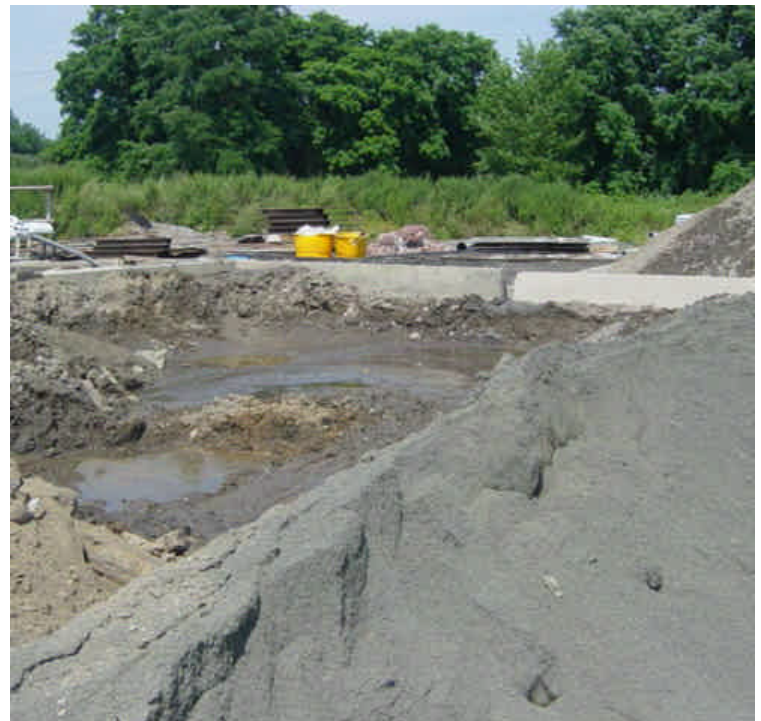
Frac tank washout water has been emptied into a containment area within the Kings Highway laydown yard. The soil berm was adequately containing the material in preparation for disposal.
