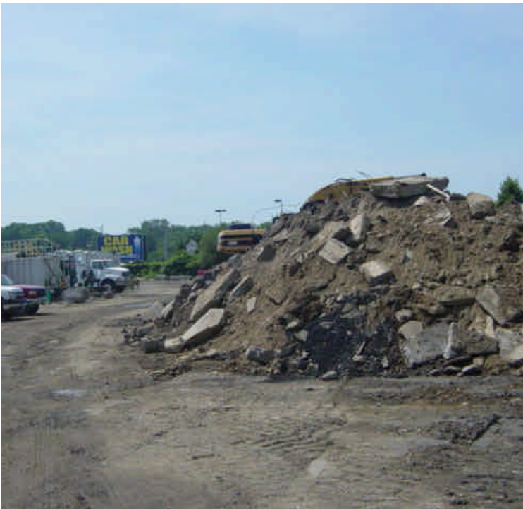
Debris pile in the Kings Highway yard has grown considerably since the previous inspection. Continue to keep material contained until it can be removed.
