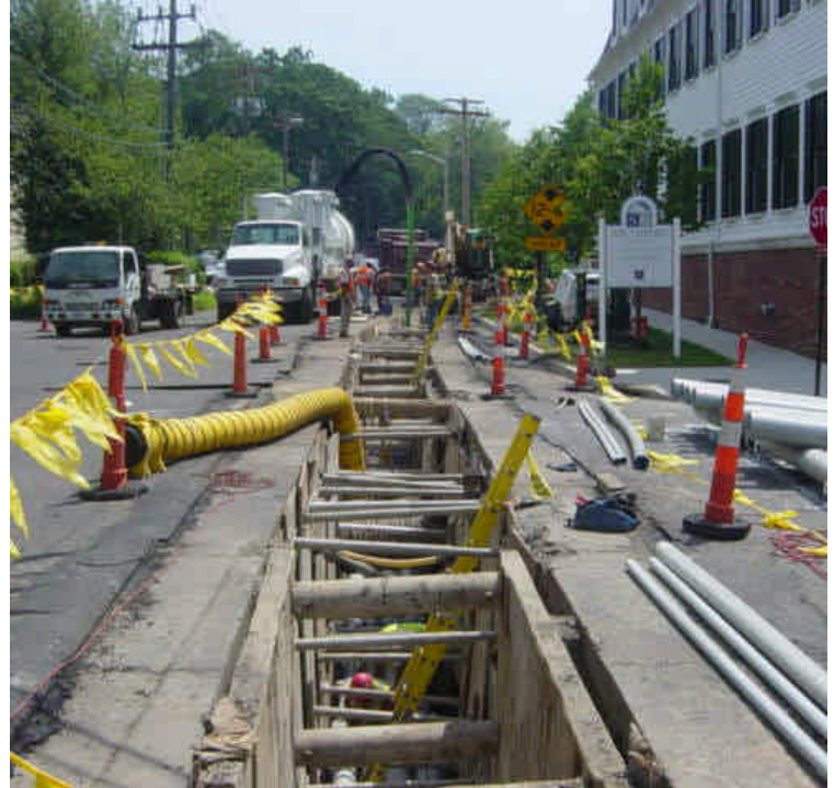
Trenching continues near sta. #468. A vac truck was on site to dewater the trench. Conduit was also being installed in some areas.
