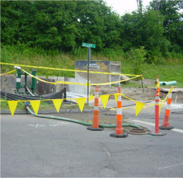
Gravel and sediment has accumulated along the curb line near sta. #647. Crews were later observed sweeping the area.
