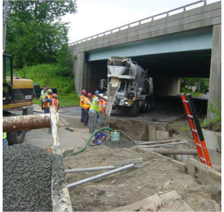
The area near sta. #719 has been partially backfilled. Minor tracking was observed along the edge of the trench.
