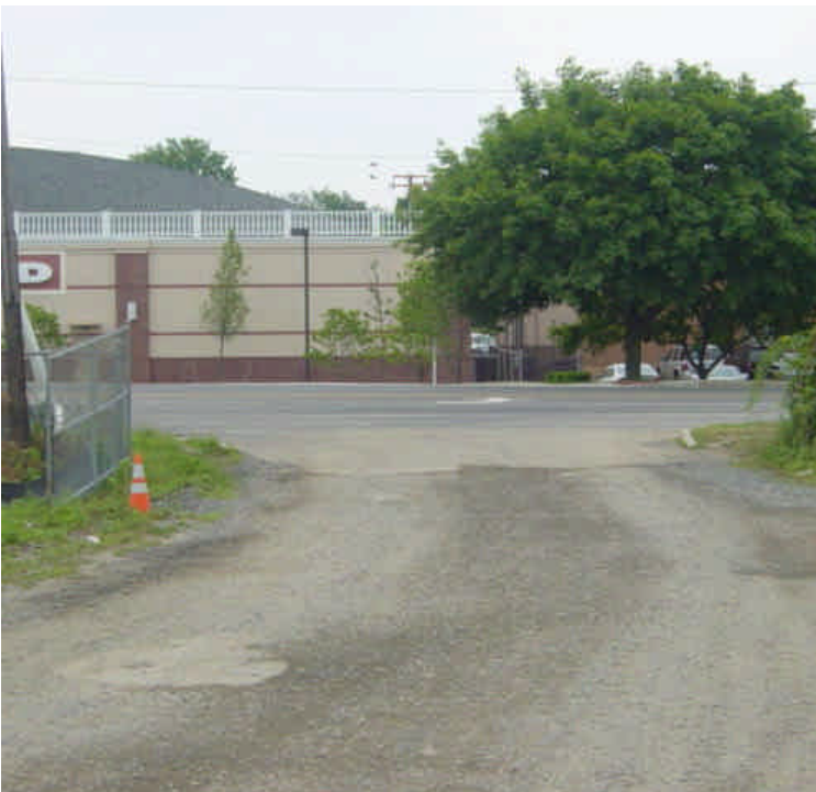
Minor tracking was observed near the entrance to the Kings Highway laydown yard. Sweep as needed.
