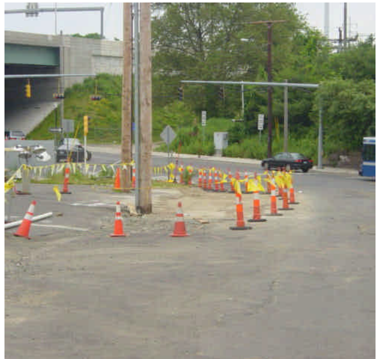
The work area near the intersection of Railroad Ave and Fairfield Ave (sta #719-720) has been backfilled with process material. Cones remain in place to prevent vehicle from pulling off road and creating ruts. Minor tracking was observed near the edge of the trench. Sweep as needed.
