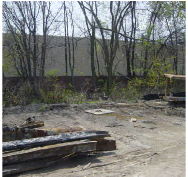
A small section of silt fence needs repair along the perimeter of the Kings Highway lay down yard.
