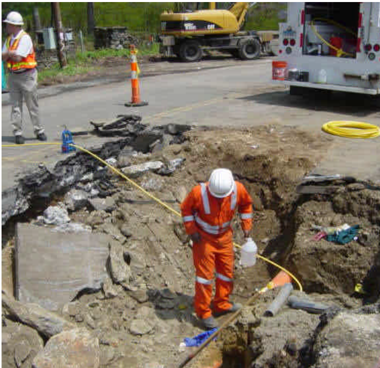
While trenching near sta. #474, a gas line was ruptured. The gas company responded to repair the broken line and there were no injuries reported.
