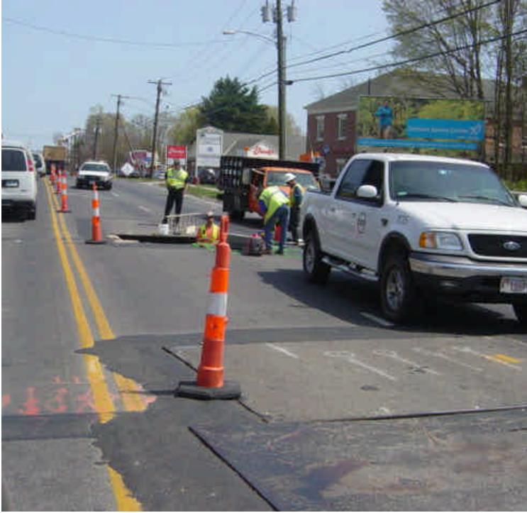
Utility work was ongoing at the bridge over Sasco Creek near sta. #441 in preparation to attach the conduit to the existing bridge structure.
