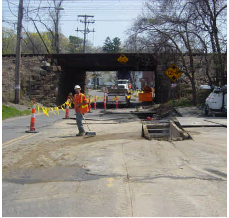
Trenching activities continue near sta. #477-478. Crews were observed sweeping the roadway in an effort to reduce sediment tracking.
