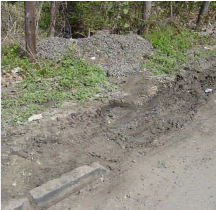
Heavy ruts were observed near the drainage swale at sta. #480. A pile of crushed stone has been placed near the edge of the swale and should be spread over the exposed soil to stabilize the area. Repair the curbing when feasible.
