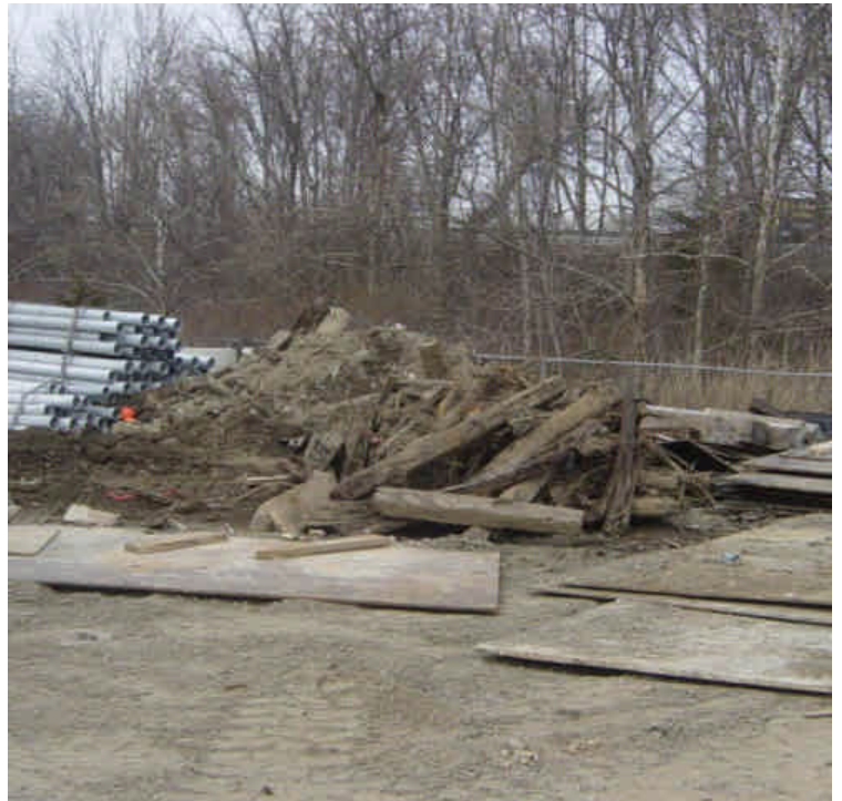
Debris materials and old railroad ties, which have been stored within the Kings Highway yard, are being sorted and processed for disposal.
