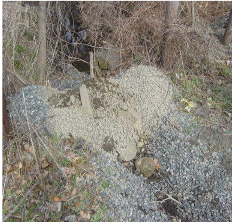
Crushed stone was placed along a drainage swale near sta. #480, to filter sediment. Some stone was inadvertently placed in the channel beyond the controls and it will need to be removed.
