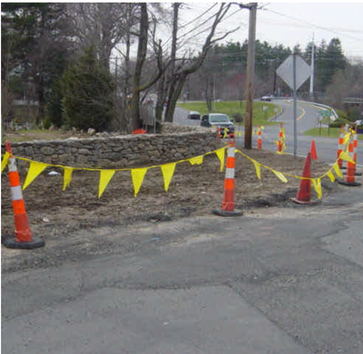
The stone wall has been reconstructed near sta. #502-503. Exposed soil still needs to be stabilized.
