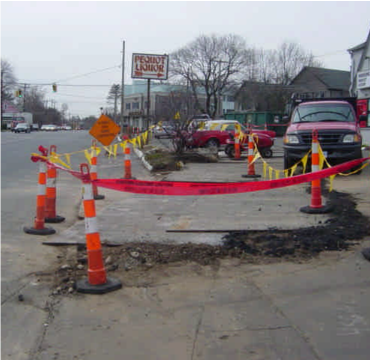
Steel plates remain over the trench near sta. #454-456 as vault tie-in work is underway.
