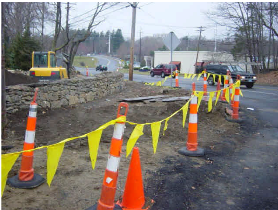
The stone wall is being reconstructed near sta. #502-503. No active work was occurring at the time of the inspection. Exposed soils around the wall need to be either temporarily stabilized or permanently restored.
