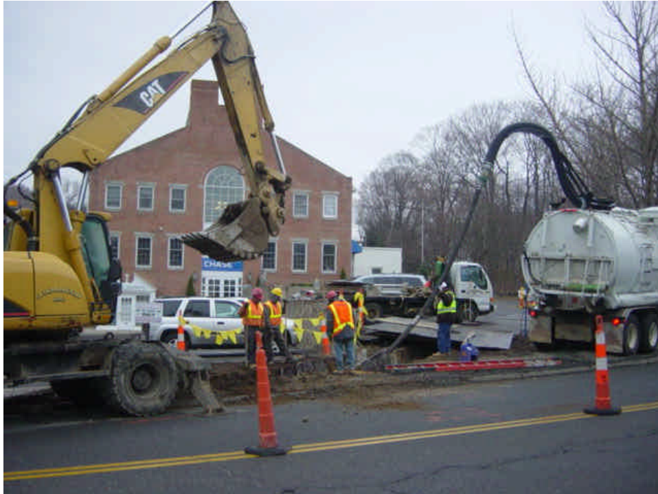
Trenching activities continue near sta. #482-483. Dewatering was ongoing at the time of the inspection and water appeared to be handled appropriately.
