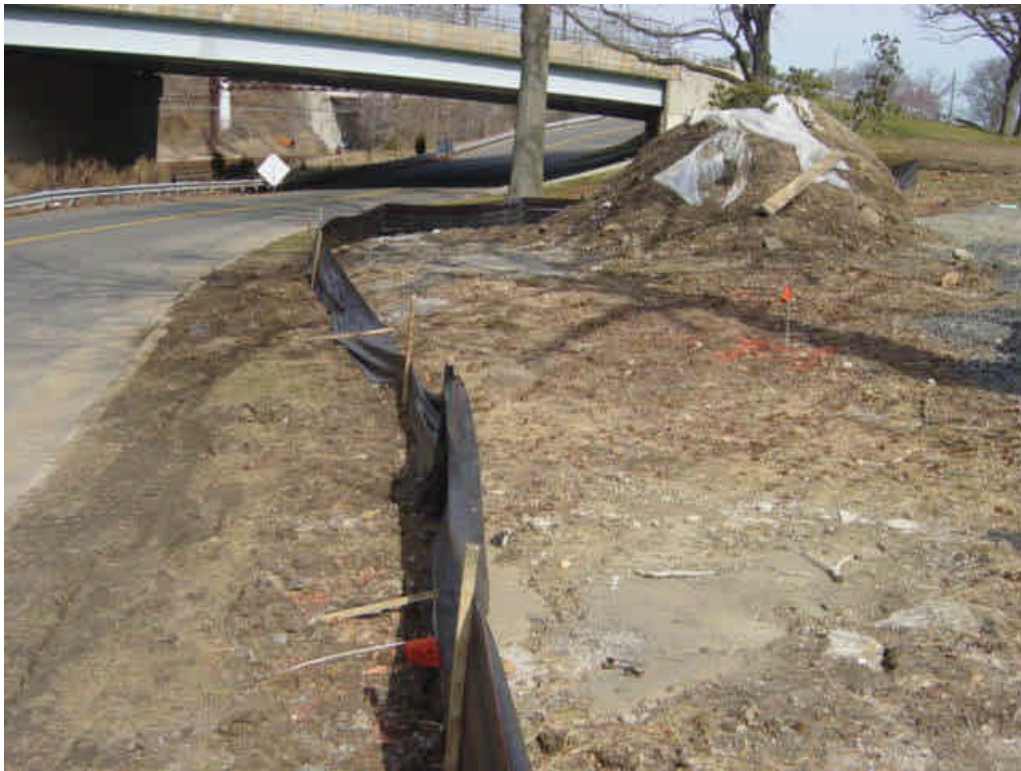
Multiple concrete washouts were observed along the median near sta. #495. The areas were contained within erosion controls, but a single, lined location should be designated for future washouts to minimize unnecessary impacts.
