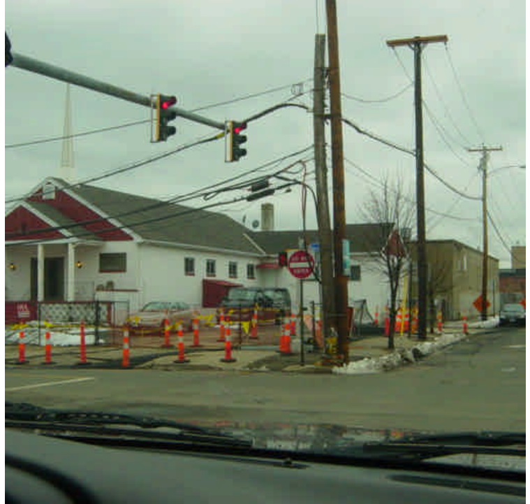
Trenching has been completed at stations 799-800. Steel plates were in place while no active work was in progress.
