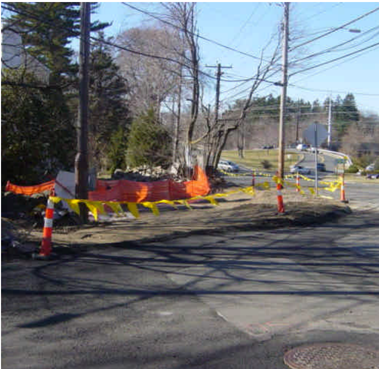
Work continues near sta. #502-503. A temporary bituminous curb has been installed and steel plates remain in the parking lot area across the street.
