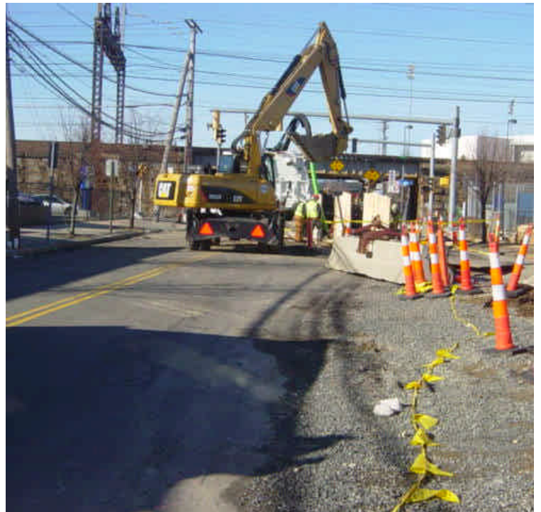
Trenching and backfilling activities continue near sta. #799. Some remnants/pebbles of temporary cold-patch material were observed in the area of the work zone along the curb and sidewalk.
