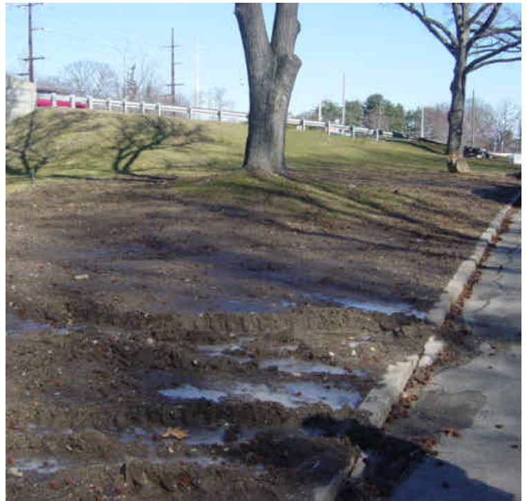
Rutted area along Pequot Ave. near sta. #495 has been re-graded to remove the ruts. A minor amount of sediment remains along the roadway and curb line. Mulch should be placed on exposed soil.
