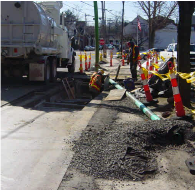
Trenching activities continue along Pequot Ave. near sta. #482 to 485. A temporary diversion drain has been installed to facilitate drainage along the roadway during construction.
