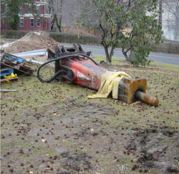
A hammer/breaker attachment containing hydraulic fluid was being stored on the median near sta. #495 without proper, proactive secondary containment.
