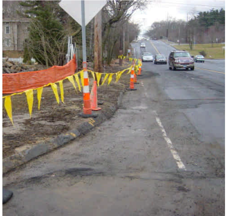
Work continues near sta. #502-503. The roadway appears to have been recently swept. However, a minor amount of sediment remained along the curb line.
