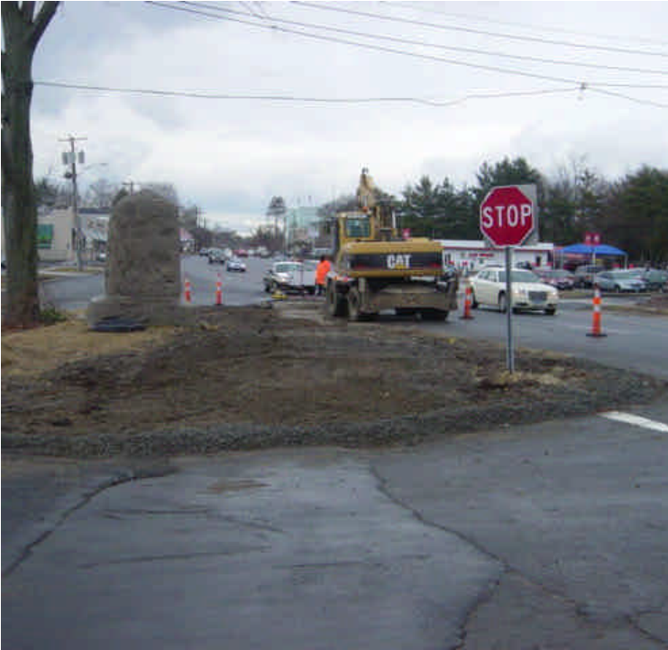
Crushed stone has been placed around the edge of the median to form a temporary curb near sta. #461.
