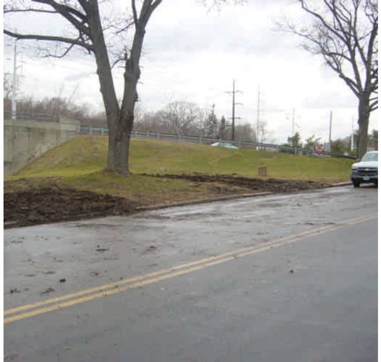
Equipment is being stored on the median near sta. #496 to 497, which has resulted in large ruts in a previously undisturbed area. Sediment was also observed on the roadway and along the curb line.
