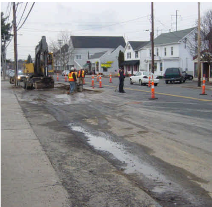
Trenching and backfill operations continue at sta. #535-536. Sediment tracking and some run-off was observed along the roadway.
