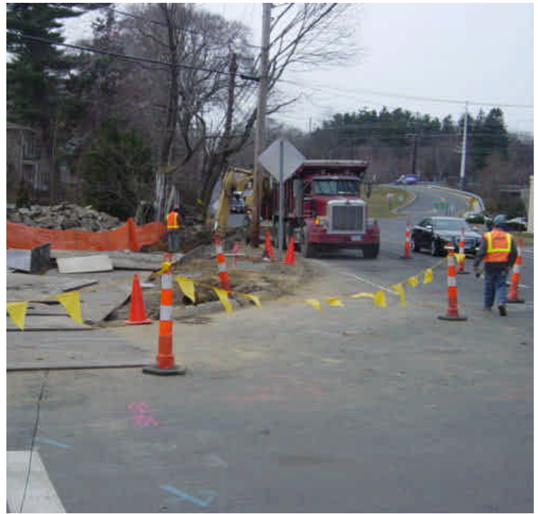
Trenching activities continue at stations #503-504, a portion of a stone wall has been removed. The stones have been placed in the adjacent homeowner's back yard until the wall can be restored.
