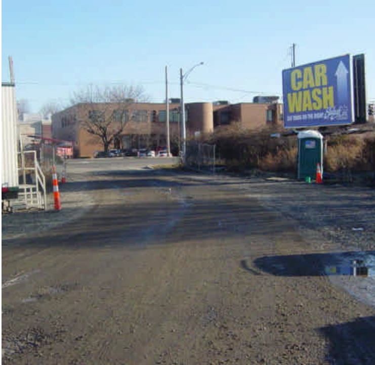
At the Kings Highway laydown yard, crushed stone has been used to temporarily stabilized the entrance but minor sediment tracking was observed on the roadway. The debris has also been removed from around the silt fence at the entrance.
