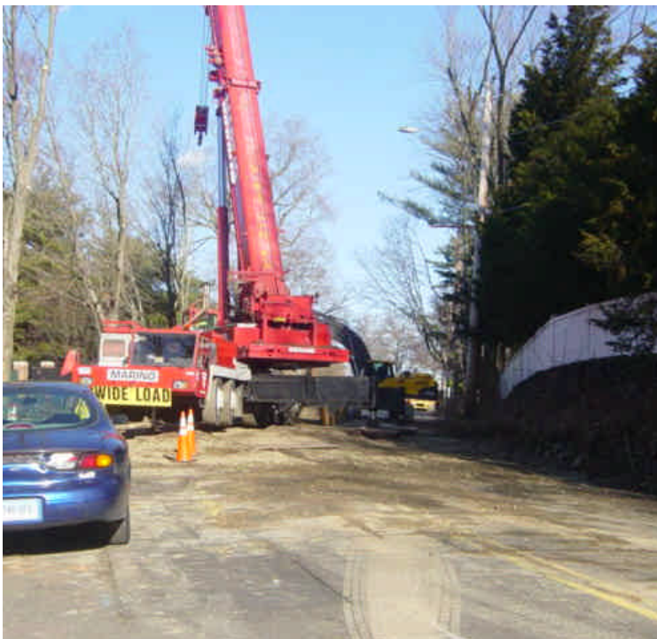
Near station #490, a crane was setting vault 29 into place on Pequot Avenue. Steel plates and sediment tracking were observed in the roadway here. Sweep all sediment before the end of the work day.
