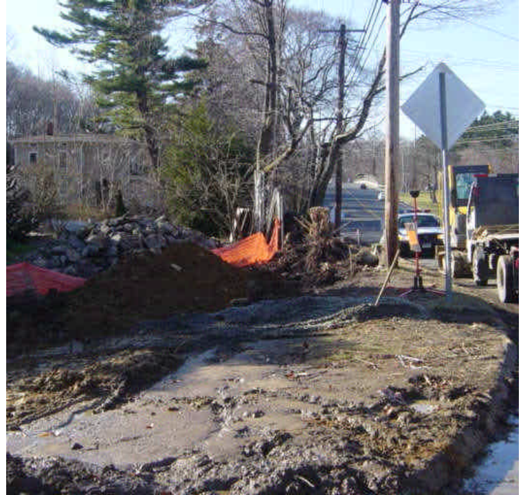
At stations #503-504, a portion of a stone wall has been removed. The stones have been placed in the adjacent homeowner's back yard until the work is complete. The silt fence surrounding a soil stockpile next to the roadway has collapsed.
