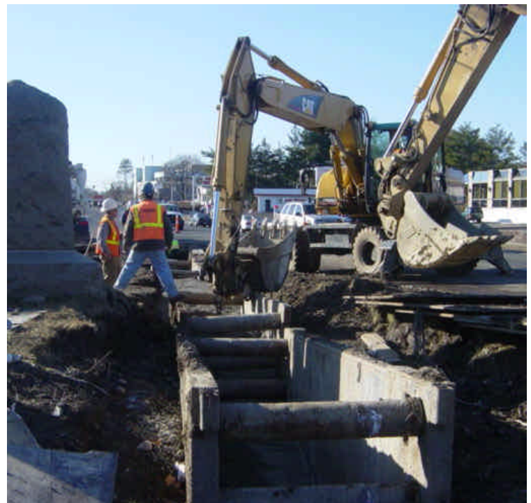
At stations #462-464, trenches were being filled. Ruts and sediment tracking need attention here. There was slurry being spilled on the ground during the inspection. Sweep the roadway at the end of the workday and attend to the slurry.
