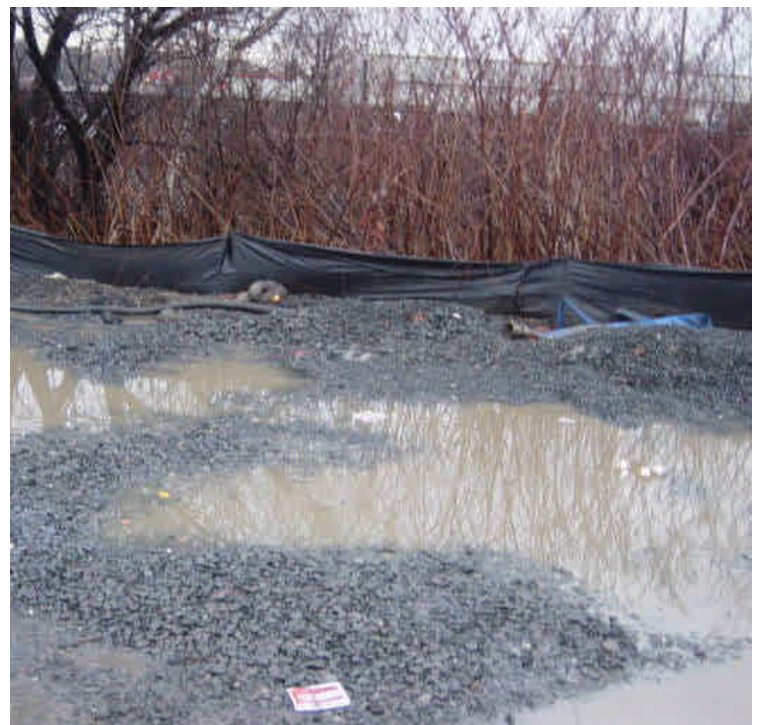
Silt fence was present around the edge of the Kings Highway laydown yard. Turbidity was observed in puddles contained to site during a rain event. No sediment tracking was observed at the entrance to the laydown yard. Piles of stone had been created during snow clearing and should be spread within the yard.
