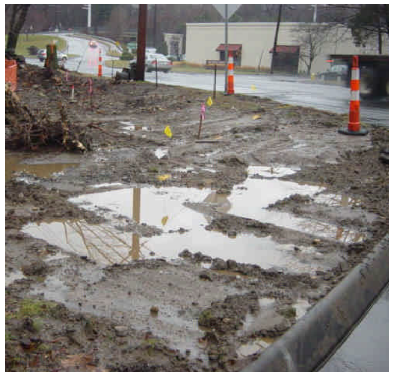
The area near station #503-504 has been grubbed to prepare for trenching. A pile of soil was contained with silt fence. No sediment tracking was observed in this area.
