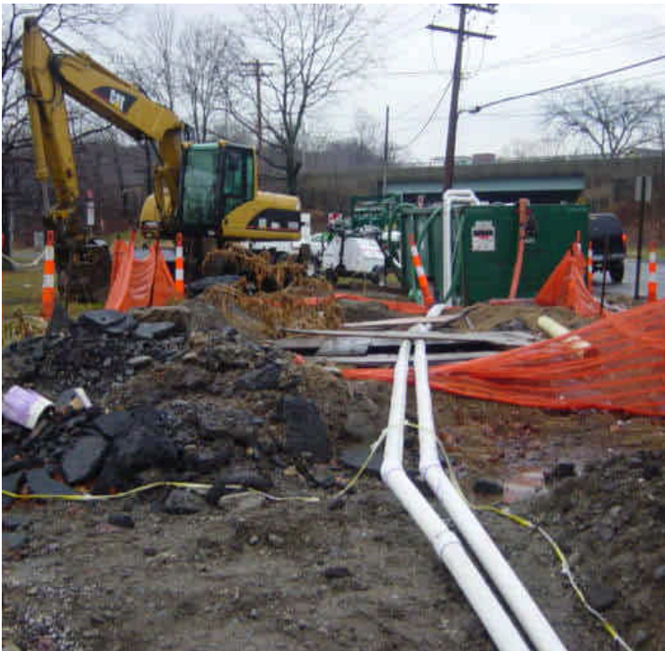
Dewatering from the frac tank was taking place near station #462-464. Clear water was observed overflowing from the containment tank onto the soil surface. This caused minor amounts of sedimentation to flow onto the roadway.
