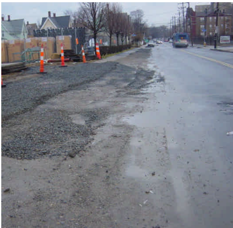
Exposed soil along the shoulder near sta. #801-803 had been partially covered with crushed stone. Further temporary stabilization should occur and roadway should be swept as needed.
