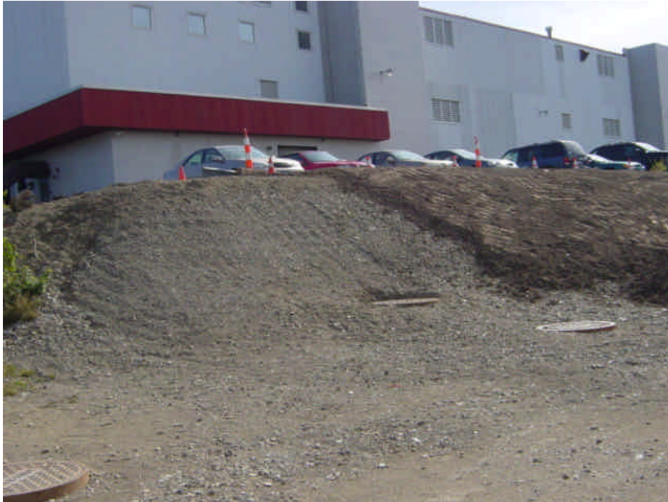
New topsoil had been applied to a portion of the slope near sta. #1080 last week. Complete the application and ensure that soil is stabilized with mulch as soon as feasible.
