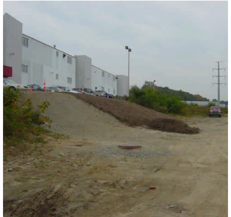
New topsoil was being applied to the slope near sta. #1080. Ensure that soil is stabilized with mulch as soon as feasible.
