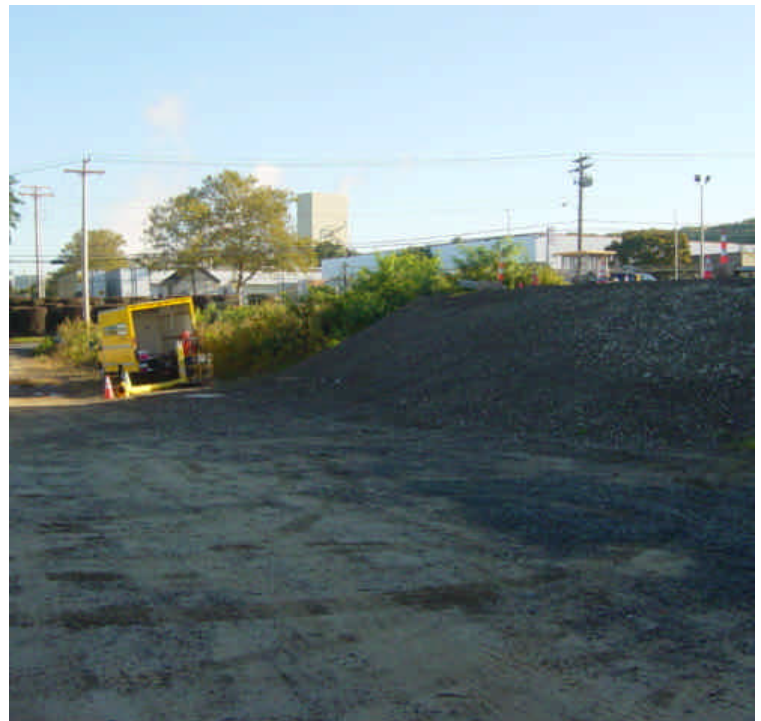
Slope near sta. #1080 remains exposed. The area has been this way for several weeks and needs to be stabilized. Electrical contractor was also on-site at vault #5.
