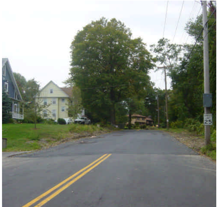
Area near vault #3 has been resurfaced as part of final restoration. Exposed process material at the base of the adjacent lawn should be covered in topsoil and seeded.
