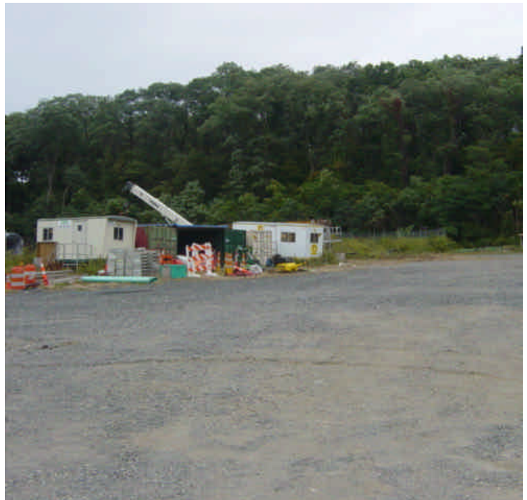
Equipment continues to demobilize from the Shelland Street lay-down yard as work is concluding
