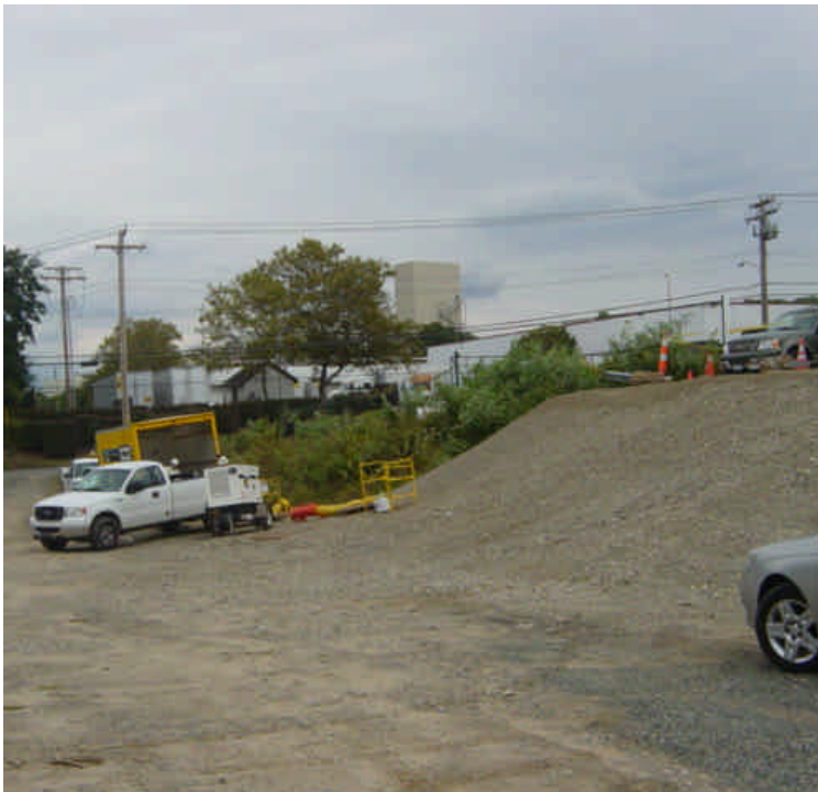
Electrical contractor was on site near sta. #1080 performing work at vault #5. The exposed slope needs final stabilization.
