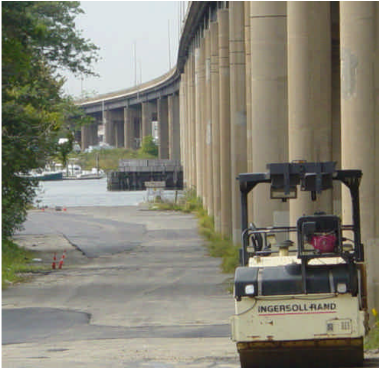
Area near sta. #1015-1020 was being paved at the time of the inspection. Once completed, the area will be fully restored.
