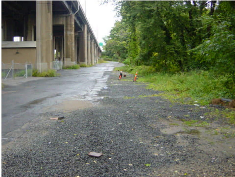
Area near sta. #1015-1020 remains stable and is temporarily backfilled with crushed stone. The area is waiting to be paved.
