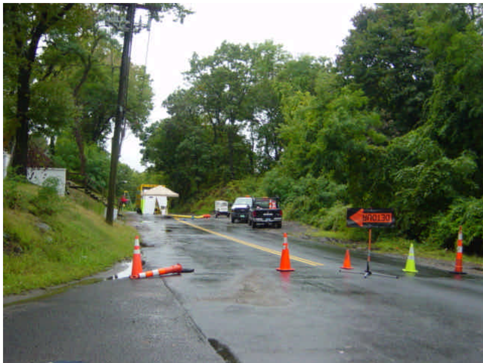
Electrical contractor was on site near sta. #1031 performing work at the vault.
