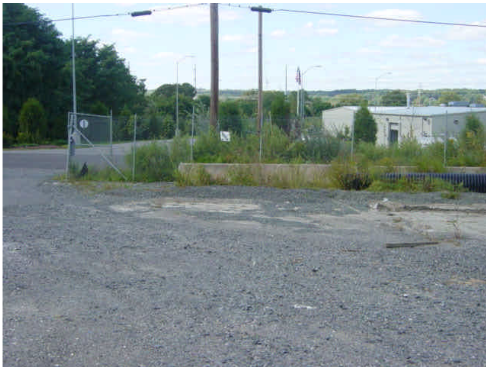
Accumulated sediment remains contained near the entrance to the Shelland Street yard. Equipment is being demobilized as work is concluding.
