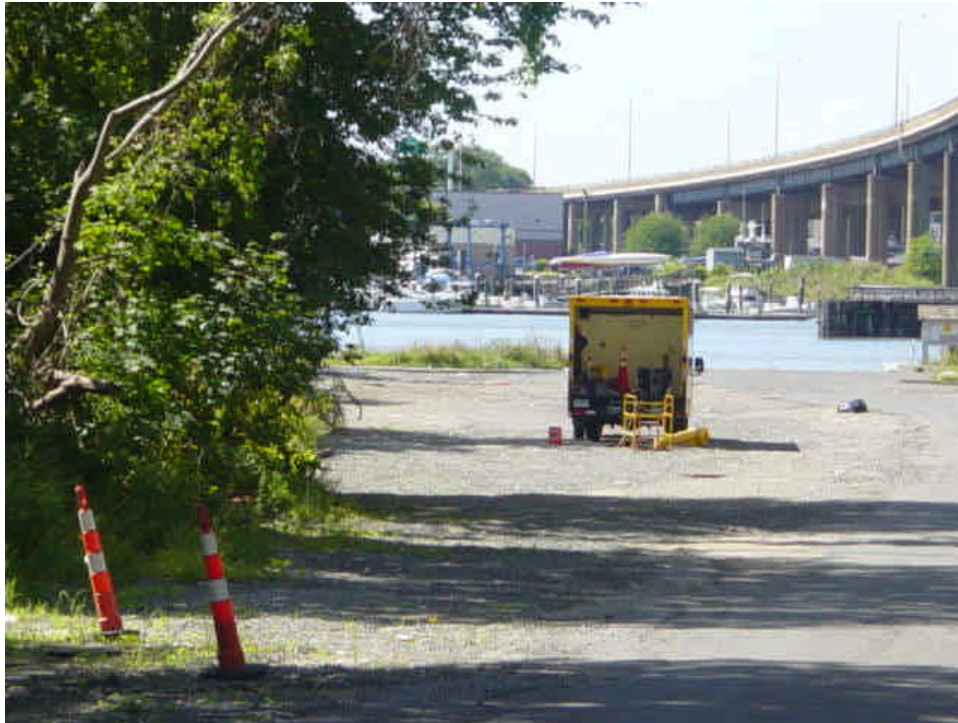
Electrical contractor was on site at vault #1.
