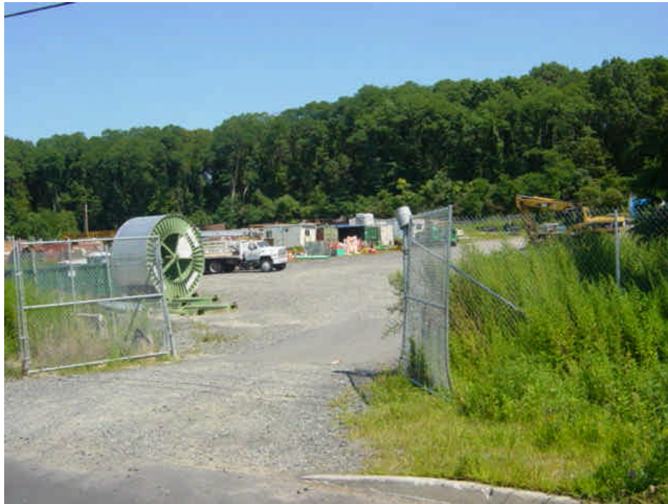
A contractor lay-down yard is located in Milford off of Shelland St. Stone is in place throughout the yard to reduce mud and subsequent tracking
