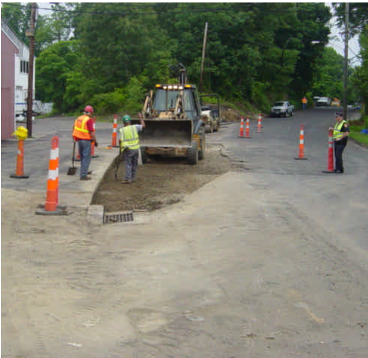
HDD tie-in work has been completed near sta. #1030. A small section was being regraded to facilitate drainage. Sediment has accumulated along the edge of the roadway near the catch basin. Controls should have been installed with the adjacent work.
