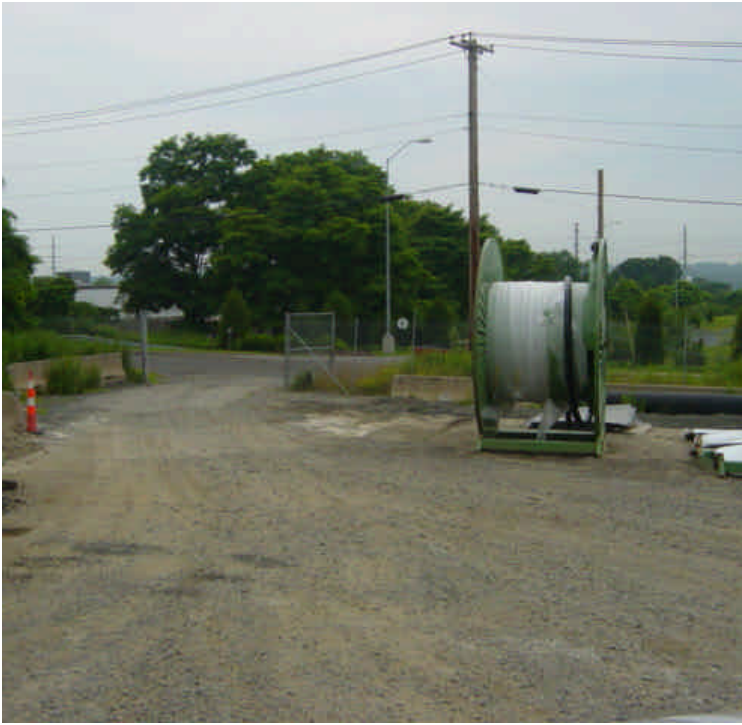
Some of the accumulated material has been removed from the stone barrier near the entrance to the Shelland St. yard.
