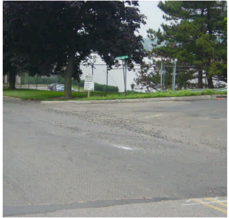
Portions of Caswell St. and Shelland St. have been milled in preparation for paving activities.
