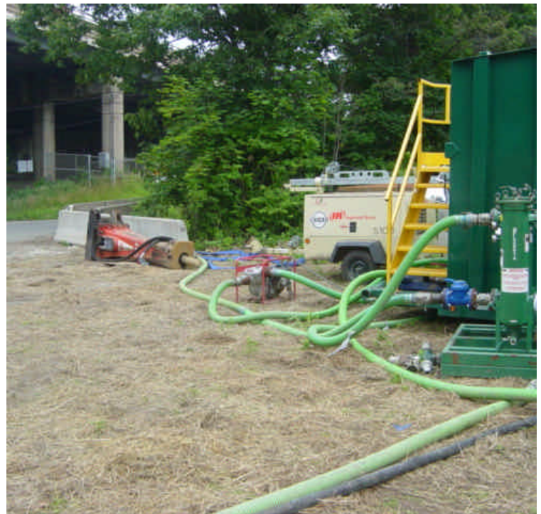
Hydraulic jacking hammer was stored near sta. #1020 without proactive secondary containment.
