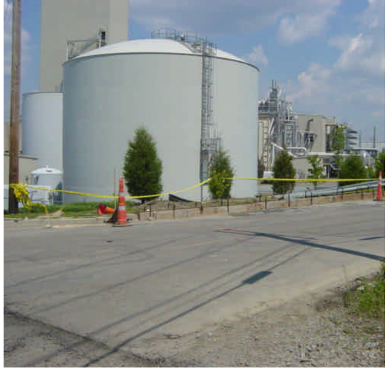
Formwork has been constructed near sta. #1095 in preparation to restore concrete curb.
