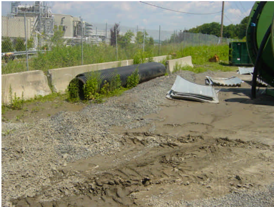
Some of the accumulated material has been removed from the stone barrier near the entrance to the Shelland Street yard.
