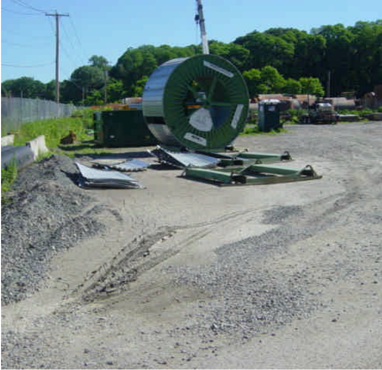
Frac tanks have been emptied out at the Shelland Street lay-down yard. Some of the material had overtopped the berm and spilled over the surface of the yard. It was contained by the stone check dam near the entrance to the yard.
