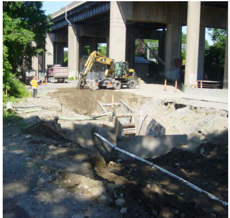
Trenching continues near sta. #1020 to connect with the HDD work. The trench was being dewatered at the time of the inspection.
