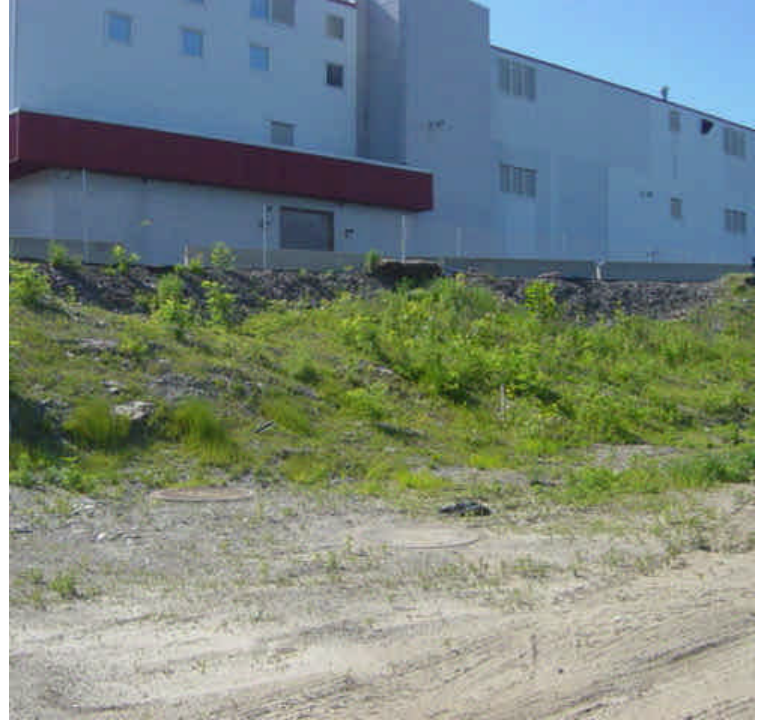
The exposed soil along the slope near sta. #1080 has naturally vegetated (approximately 90% coverage). Coordinate final restoration/planting plans with the landowner.
