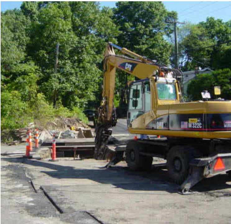
Trenching continues near sta. #1030 to connect with the HDD work. One of the circuits has already been connected.
