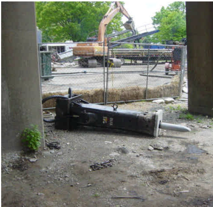
Hydraulic jacking hammer was temporarily stored along the access drive near sta. #1020 without secondary containment.
