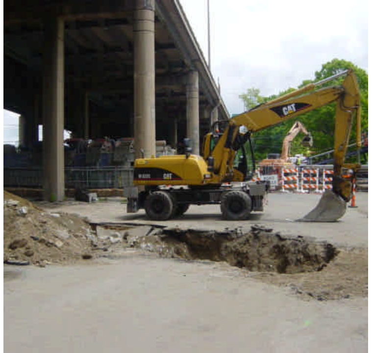
Area near sta. #1020 was being excavated to expose the conduit bank and tie-in with the HDD work.
