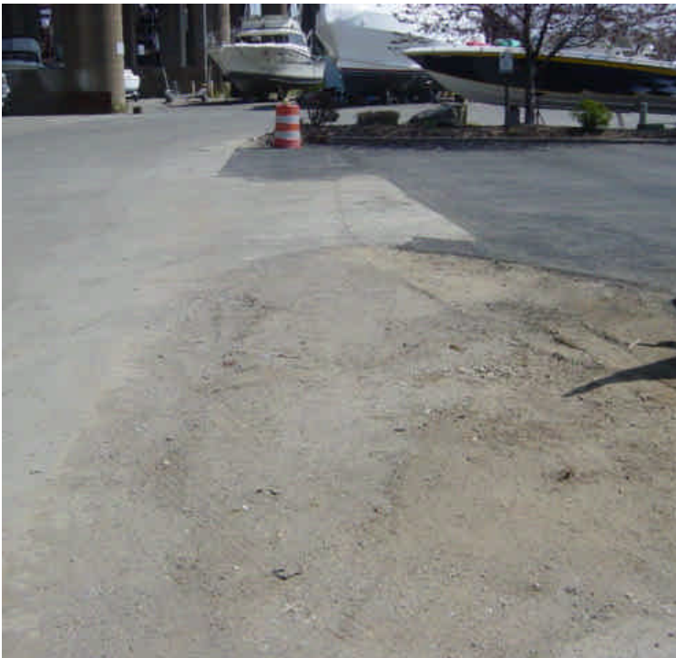
Tie-in work has been completed on the west side of the Housatonic River near sta. #999 and the area has been paved. A small section remains backfilled with soil/ processed material.
