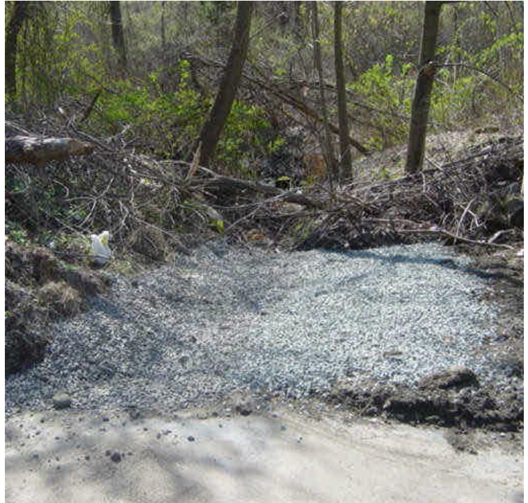
Deteriorating hay bales have been removed from the drainage swale near sta. #1017. Crushed stone has been installed to limit Sedimentation. Continue to monitor and determine if this is effective.
