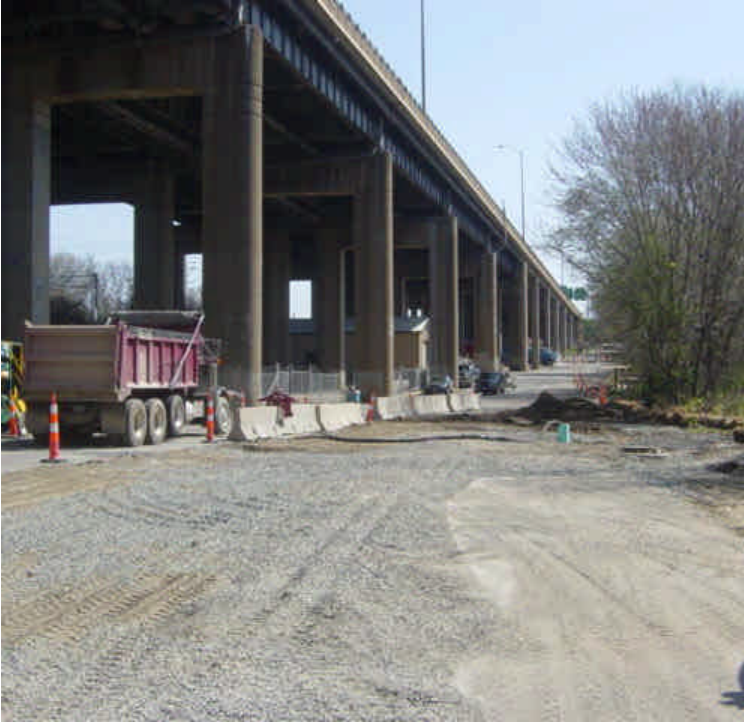
HDD work has been tied-in to the vault near sta. #1015 and the area was being backfilled with crushed stone and process material in preparation for paving.
