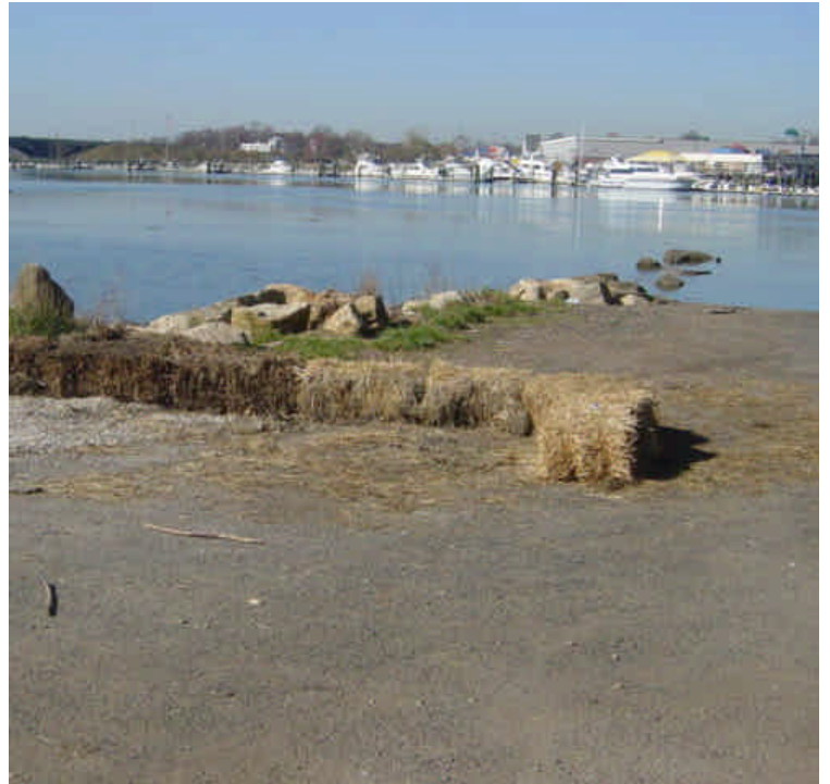
Deteriorated haybales along the bank of the Housatonic River have been replaced and reset.
