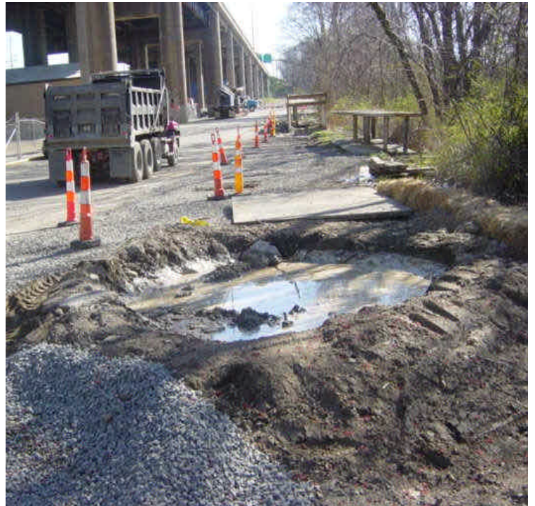
A designated concrete washout area remains in place near sta. #1018. Watch available capacity and controls here and remove material when feasible.
