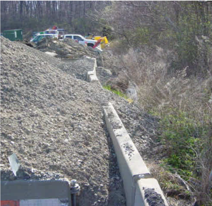
Stockpiled material has overtopped the established storage bins at the Shelland Street yard, but material remains at the perimeter controls.
