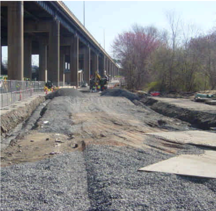
Tie-ins between the HDD work the vault near sta. #1015 are complete and the area has been partially backfilled. Handholes were being set at the time of the inspection.
