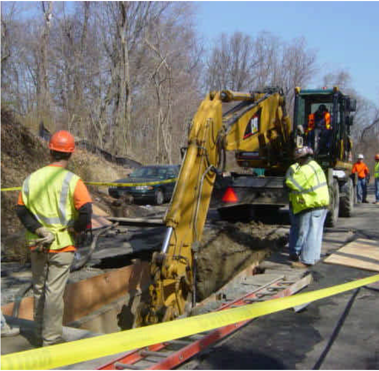
Trenching continues along Naugatuck Avenue near sta. #1031-1032. Ledge was encountered in this area.
