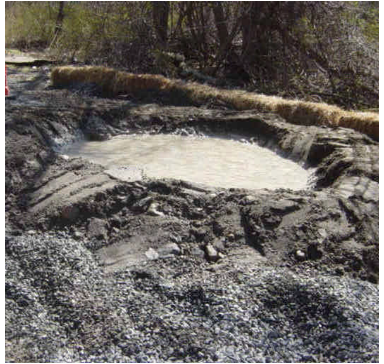
A designated concrete washout area was observed near sta. #1018. Haybales were also placed along the edge of the work zone to provide additional control/protection. Remove concrete material when feasible.
