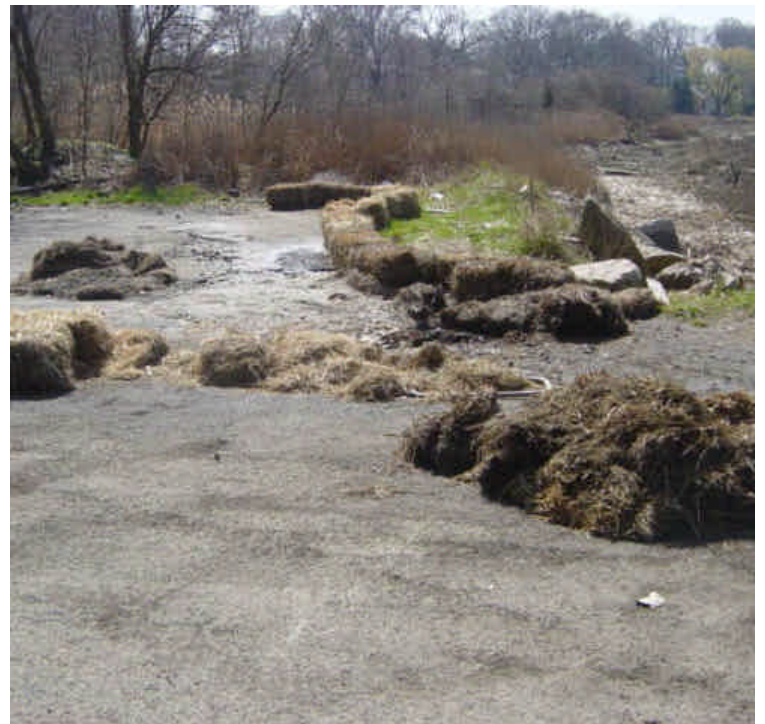
Haybales remain in place along the bank of the Housatonic River. Some of the haybales have been moved and are deteriorating. Work to restore any remaining exposed areas with their original cover (e.g. vegetation or pavement).
