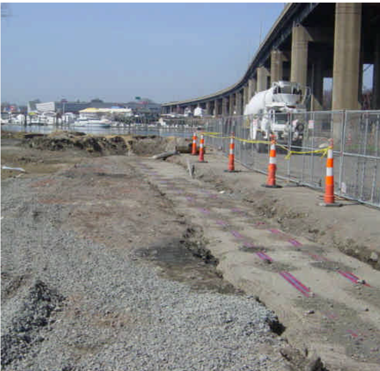
HDD work has been tied-in to the vault near sta. #1015 and the area has been partially backfilled.
