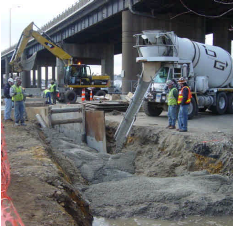
On the west side of the Housatonic River near sta. #999, vault tie-in work is complete and crews were backfill the drilling pit and trench.
