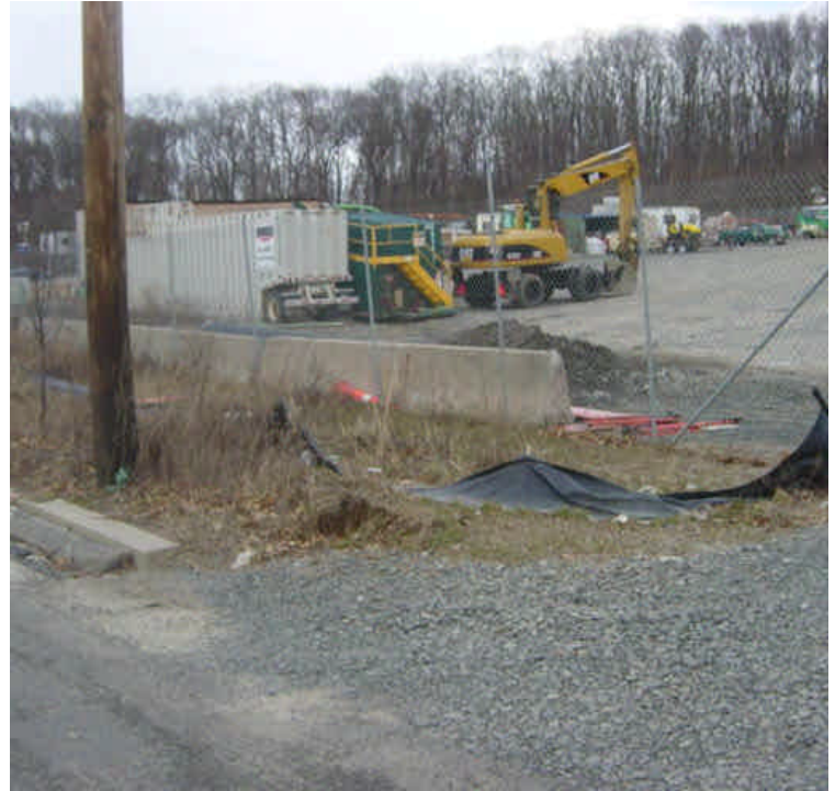
Sediment has accumulated behind the stone berm near the entrance to the Shelland Street lay down yard. A minor amount has migrated beyond the berm. The catch basin remains protected.
