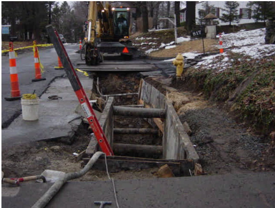
On Naugatuck Avenue, near sta. #1036-1037, trenching and dewatering were in progress. The water was being properly filtered and discharged into the sanitary sewer.
