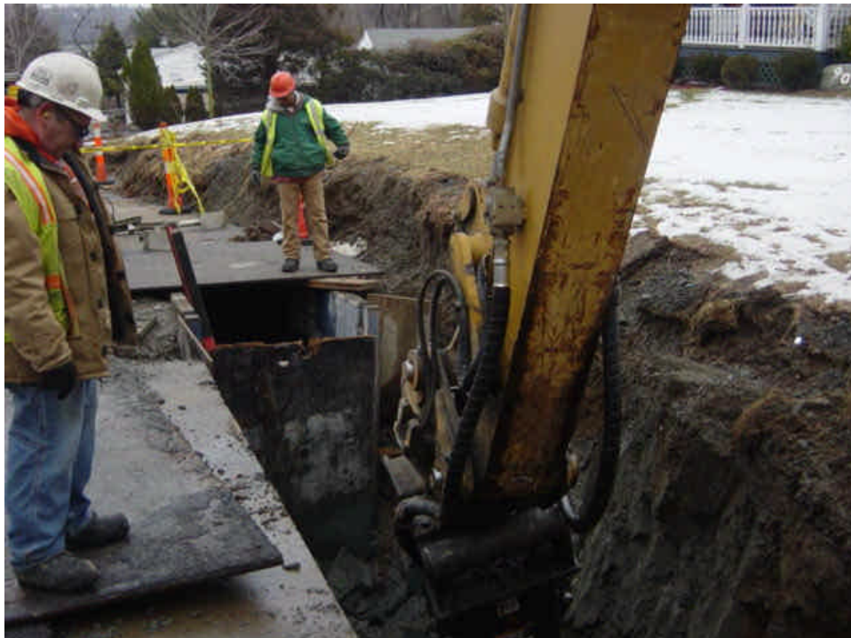
On Naugatuck Avenue, near sta. #1047-1048, the hydraulic jackhammer was being used to break through ledge.
