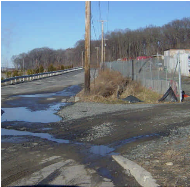
Construction entrance at the Shelland Street lay-down yard continues to function. A large pothole/ depression has formed near the entrance causing storm runoff to pond in this area.
