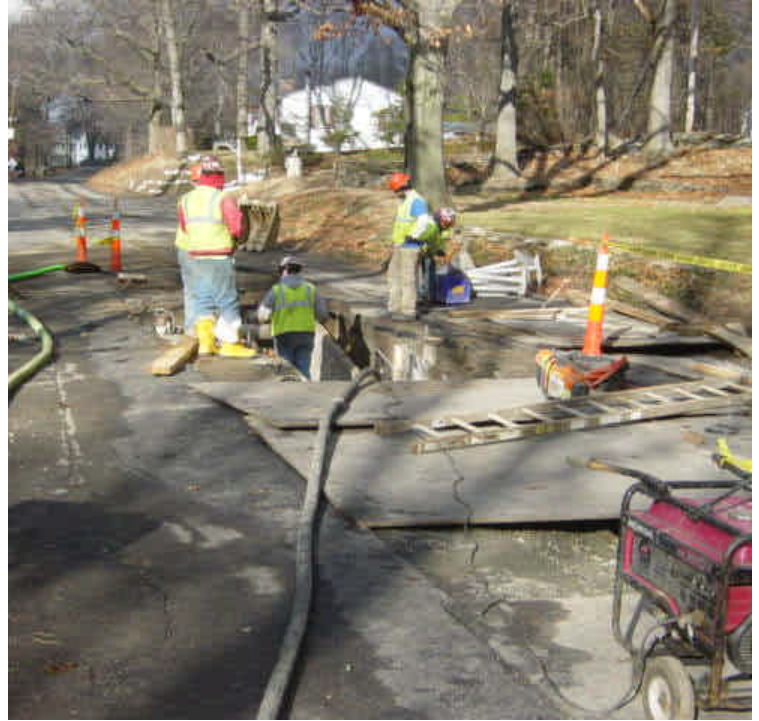
Trenching activities continue along Naugatuck Ave near sta. #1037 to 1038. At the time of the inspection, the trench was being dewatered. Water was filtered, and then discharged appropriately to a nearby sanitary sewer.
