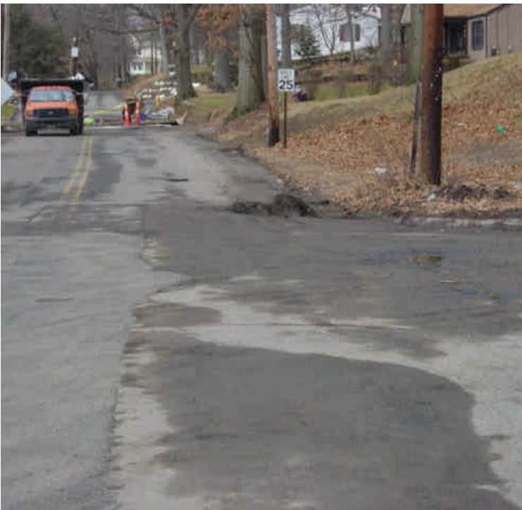
A catch basin near sta. #1034 was plugged with a large amount of sediment and debris, but was not project related. Crews removed some of the sediment to improve drainage.
