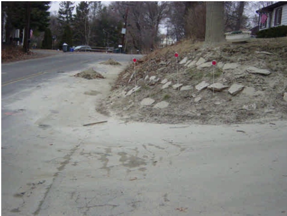
Two small piles of fine, dusty material were observed on Naugatuck Avenue near sta. #1038. The material was also observed along the adjacent driveway which appeared to have been wind blown. The source of the material/ dust was unclear and may not be project related.
