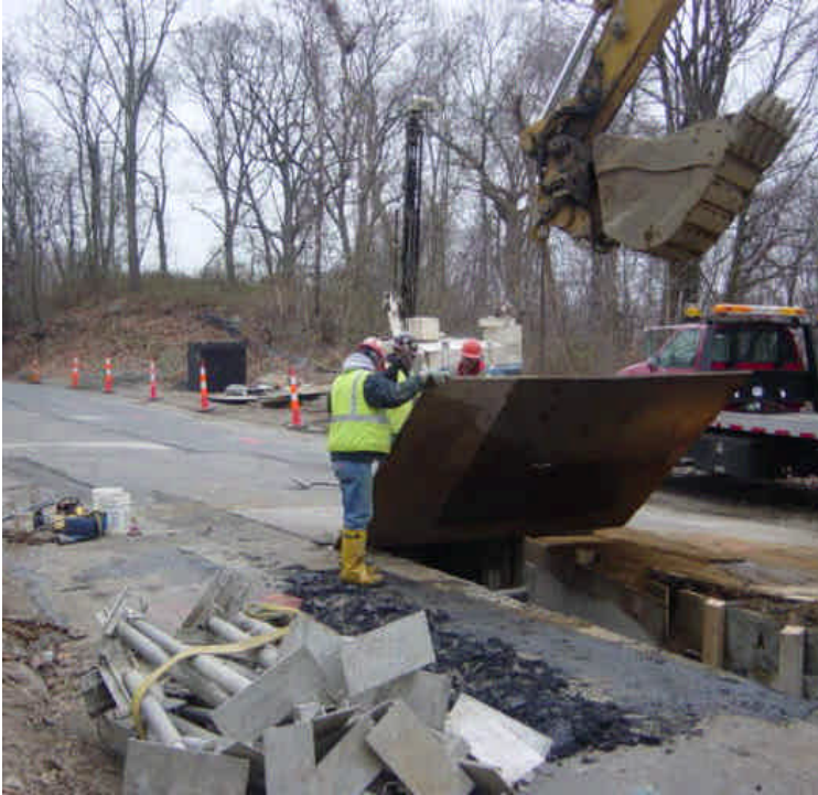
Trenching continues along Naugatuck Avenue near sta. #1032-1034. Continue to sweep roadway as sediment is generated.
