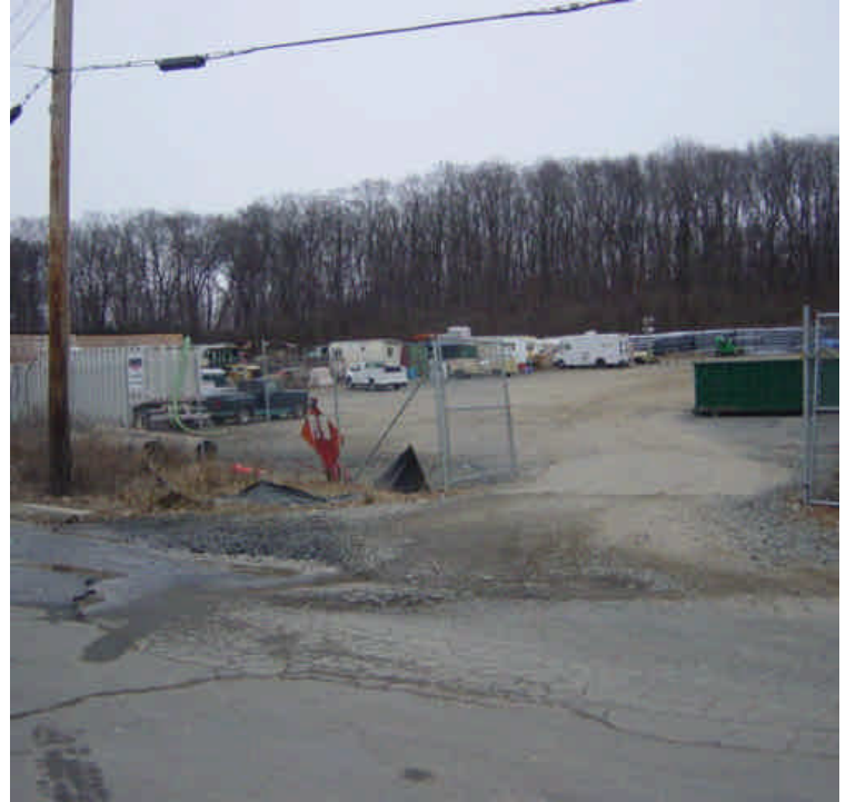
Activity has increased at the Shelland Street laydown yard as work has returned to this segment of the project.
