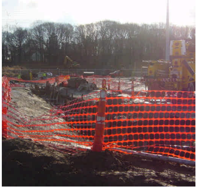
Trenching continues adjacent to the East Devon substation, between sta#1114-1119. There are large areas of exposed soil present but site is largely contained.
