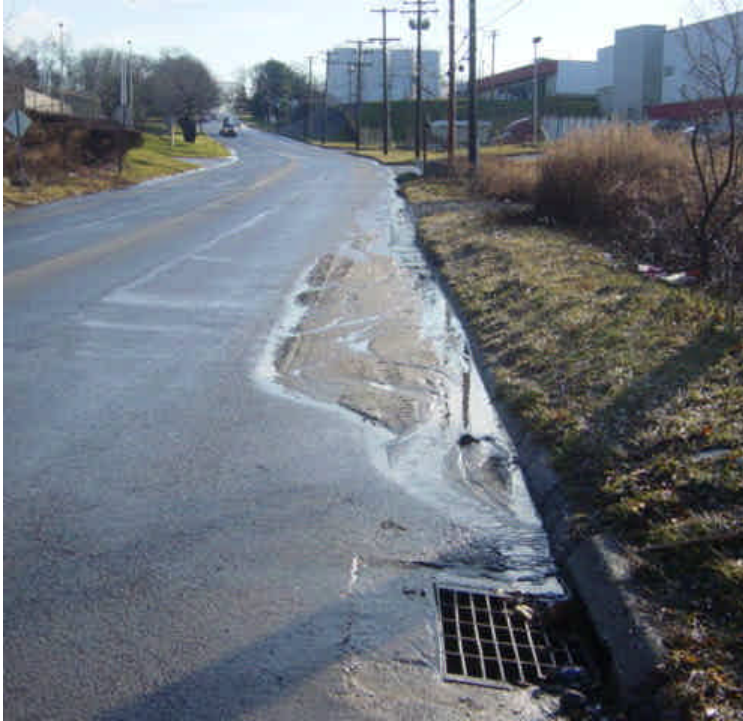
On Caswell Street, accumulated sediment remains upgradient of the protected catch basin. However this tracking is not associated with the Segment 3 work. (See overhead report 2B).
