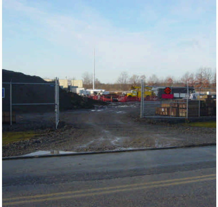
Crushed stone has been used to stabilize exposed soil at the East Devon substation entrance. Minor sediment tracking was observed on Plains Road. A very large soil stockpile is located at the entrance but this is not associated with the Segment 3 work. (See the East Devon Substation report).
