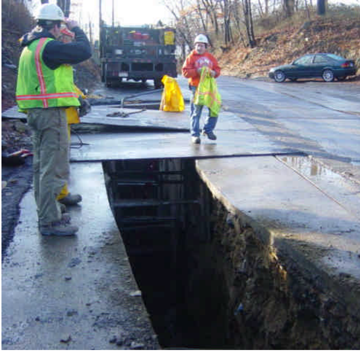
Trenching has resumed at stations #1031-1034 on Naugatuck Ave, which was closed to traffic. Water was being pumped into the empty vault for temporary storage.
