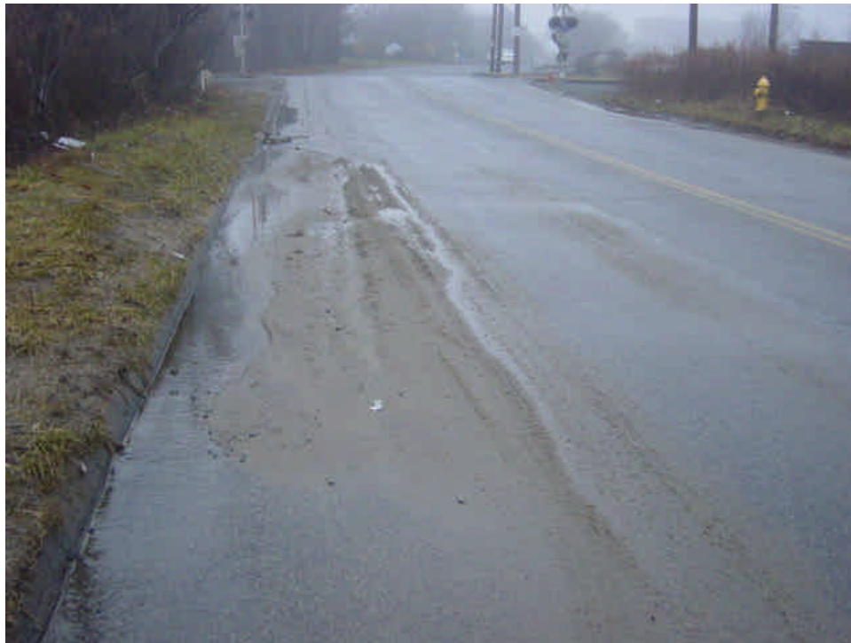
Sediment remains upgradient of the catch basin on Caswell Street. However, this tracking does not appear to be associated with the Segment 3 work. (See the overhead 2B report for more information.)
