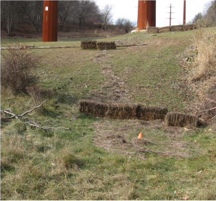
Dogburn Rd (Orange): Final stabilization has been achieved near structure #3890/24077.
