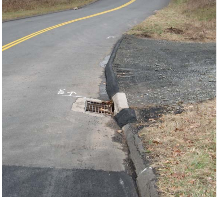
Old Ln (Hamden): A new curb has been installed at the Old Ln. ROW access. The curb will help control sediment migration to the catch basin. Catch basin protection has been removed.
