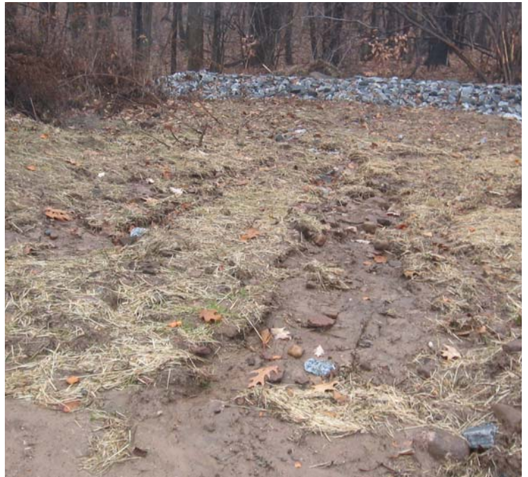
Gaylord Mtn Rd (Hamden): Runoff continues to scour exposed soils above the ROW perimeter swale.
