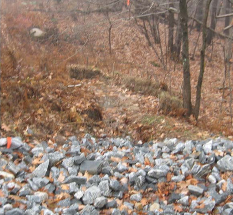
Gaylord Mtn Rd: Haybale controls continue to function near the end of the swale.
