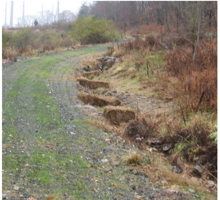
Old Ln: The access road appears to be stable at this time.
