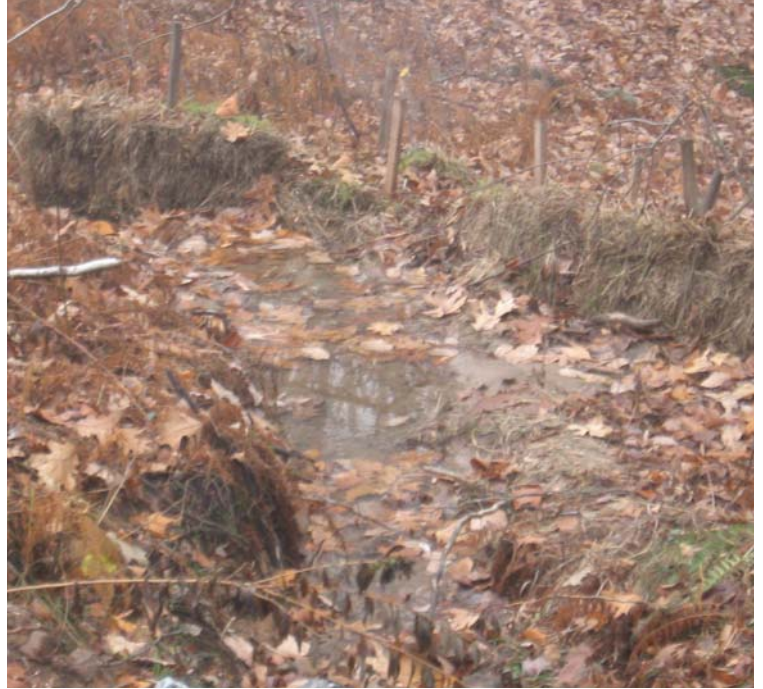
Gaylord Mtn Rd: An additional view of sediment being contained by the haybale controls.
