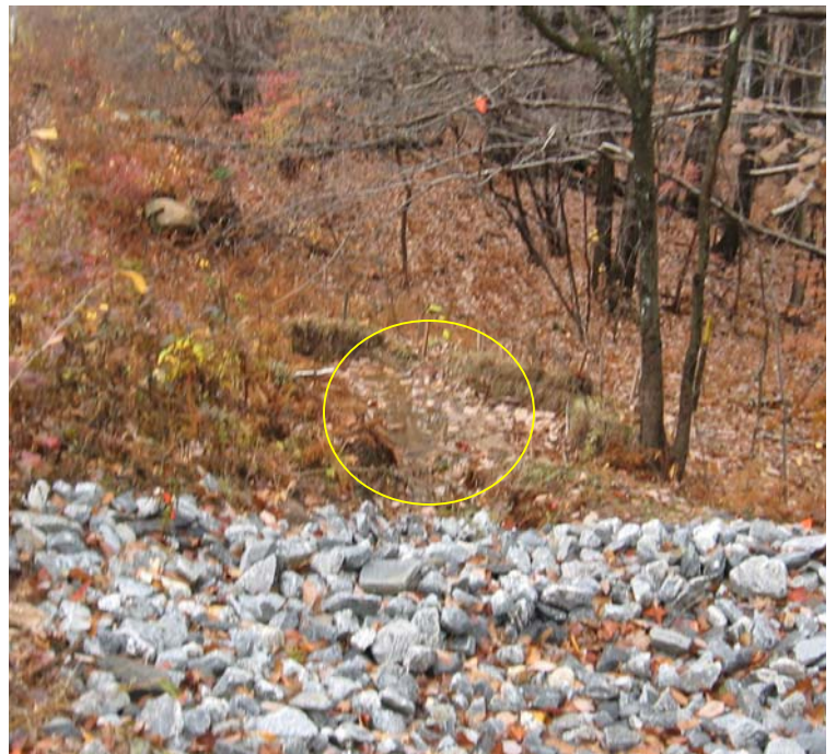
Gaylord Mtn Rd: Sediment from the scoured channels, shown in the previous photo, is accumulating at the haybale controls located at the end of the swale.
