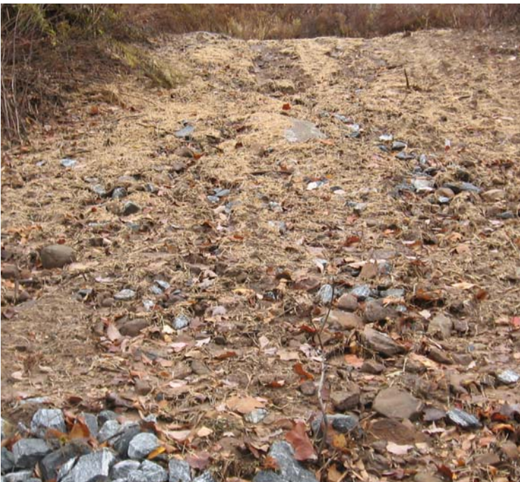
Gaylord Mtn Rd (Hamden): Some scouring has been observed where construction equipment accessed the ROW to install erosion controls. Sediment is migrating to the swale located down gradient and along the perimeter of the ROW.
