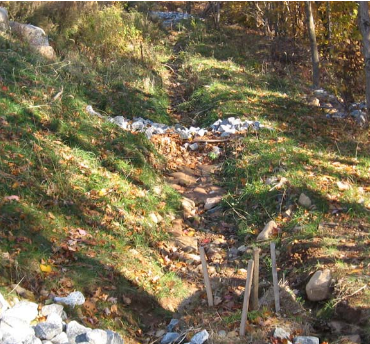
Gaylord Mtn Rd: An additional view of the controls installed within the swale.
