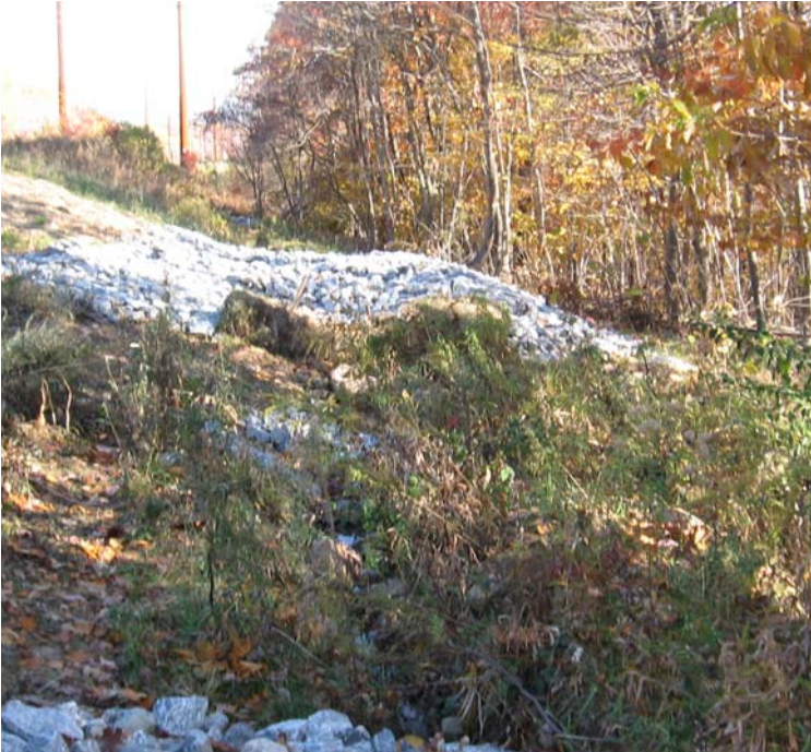
Gaylord Mtn Rd (Hamden): Stone has been added to portions of the swale located along the perimeter of the ROW.
