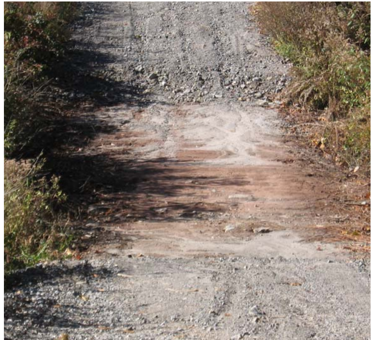
Brooksvale Ave: It appears sediment from the access road is migrating into the wetland during storm events. Additional controls are needed here.
