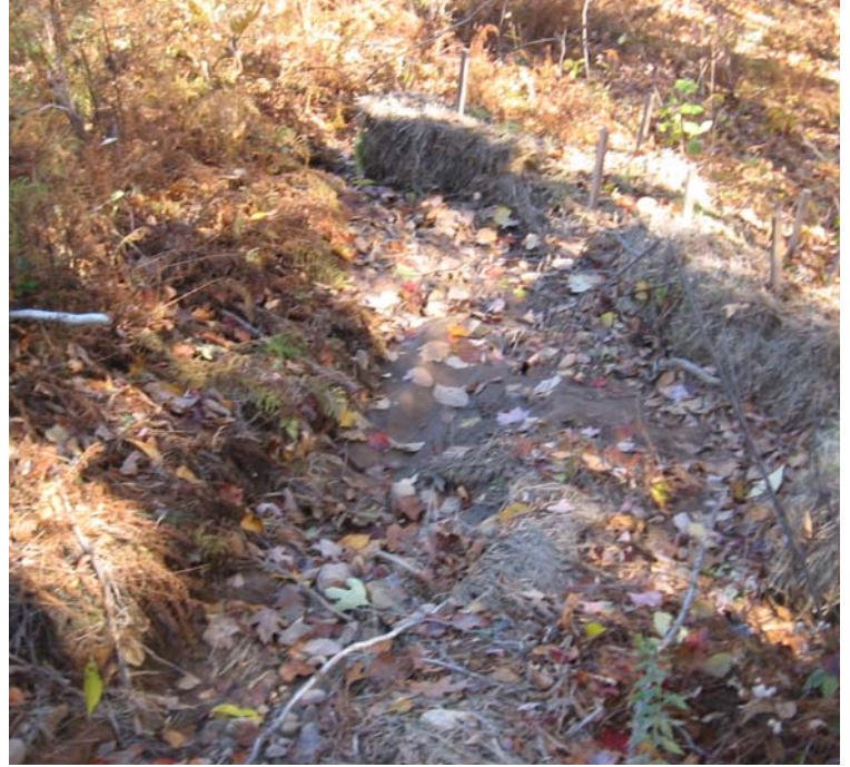
Gaylord Mtn Rd: The haybale controls at the end of the swale are helping to control sedimentation to a wetland off the ROW.
