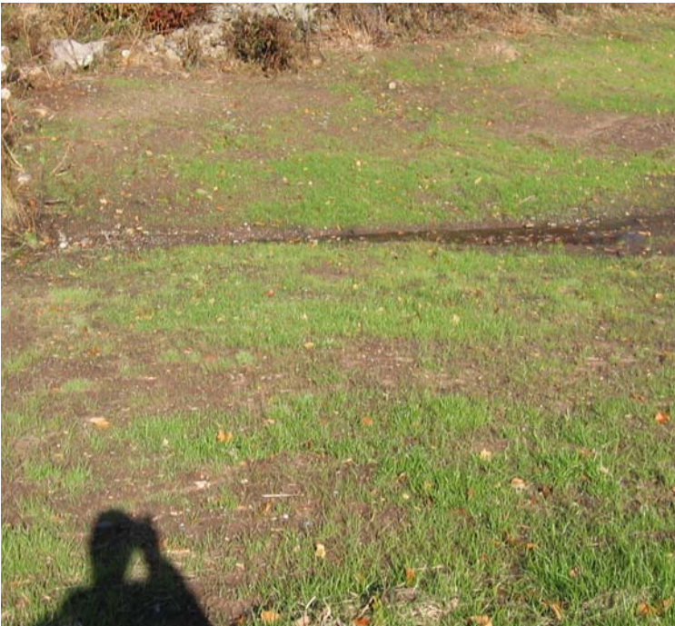
Pease Rd/JCC (Woodbridge): Vegetative growth continues within the restored access road. Haybale controls have been recommended along the watercourse here.
