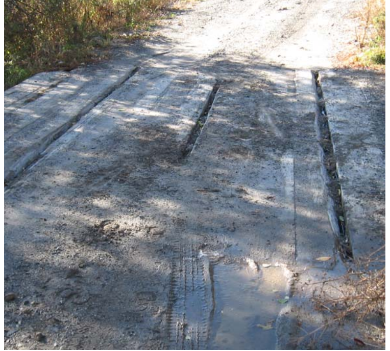
Litchfield Turnpike: Silt fence has been placed in the cracks of the timber mat crossings as a temporary sediment control.
