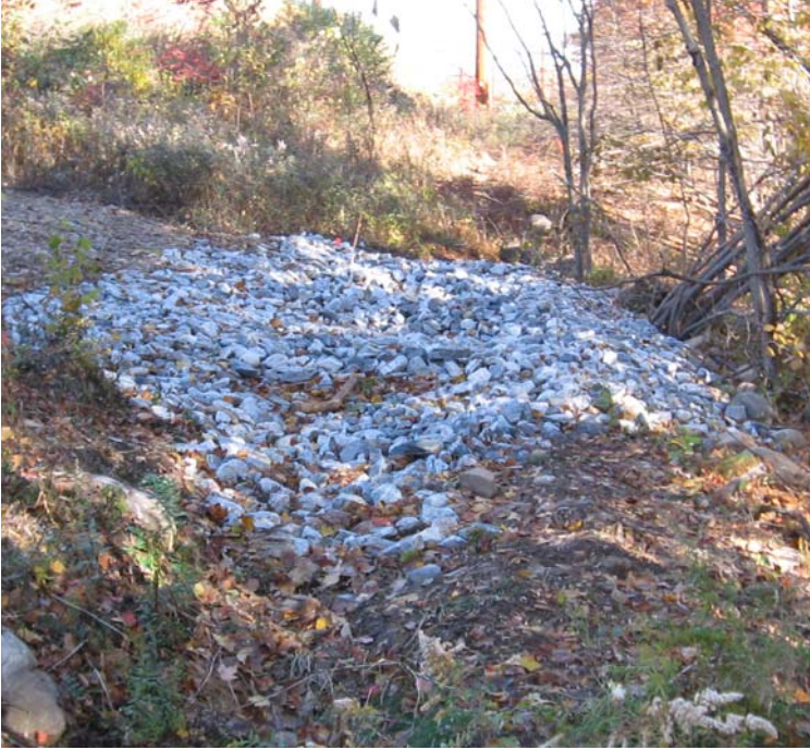
Gaylord Mtn Rd: This stone check dam is located at the end of the swale just prior to runoff leaving the ROW.
