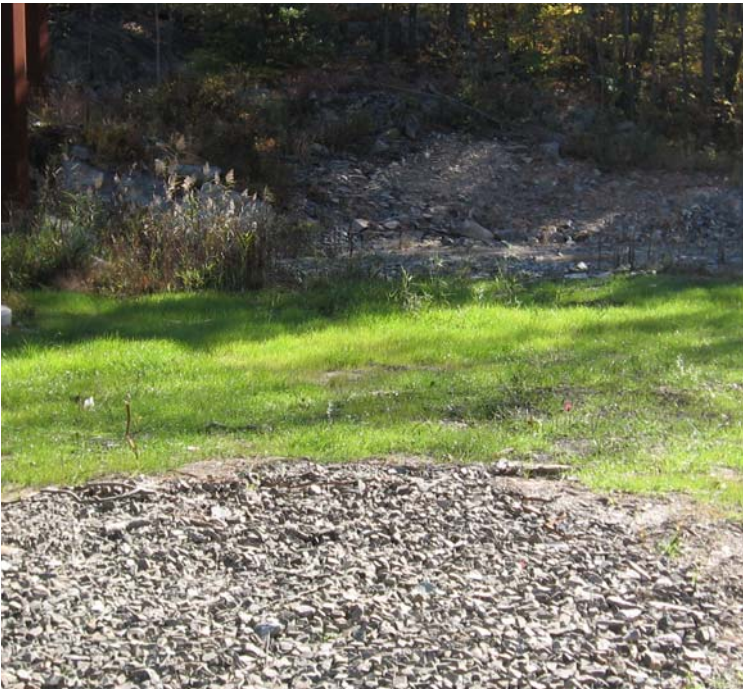
Rt 34: An additional view of the permanent access road within the wetland near structure #24072.
