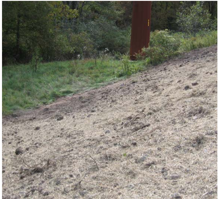
Willow St: Additional view of the crane pad restoration efforts near structures #4009/24196.
