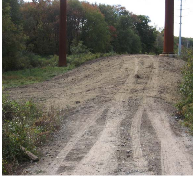
Willow St (Hamden): View of the restoration efforts here. Soils appear stable at this time.
