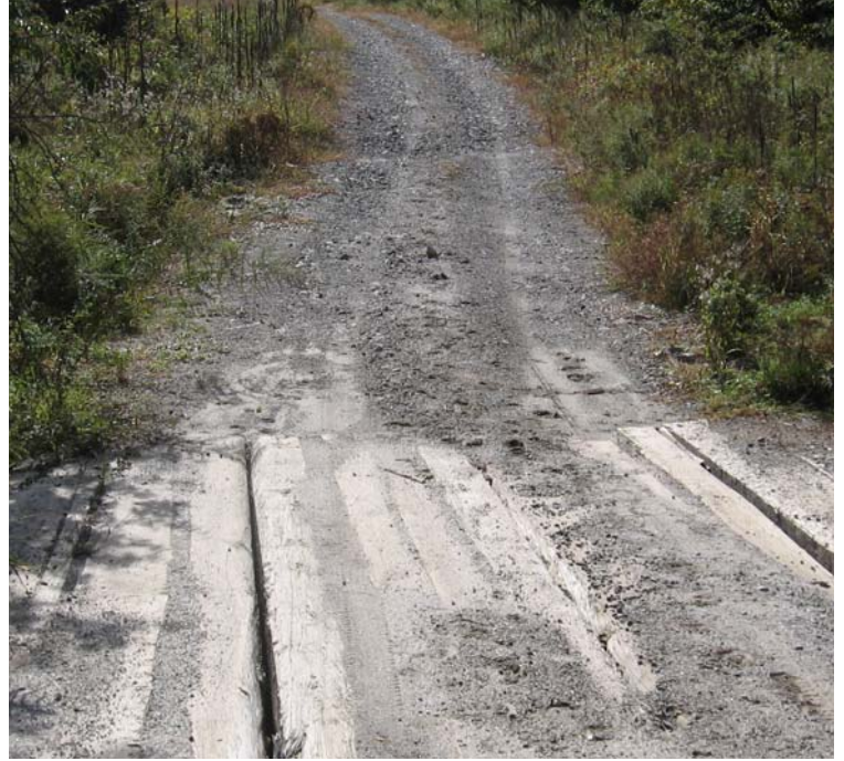
Litchfield Tpk: Sediment from the access road is migrating to the watercourse at the permanent crossings.
