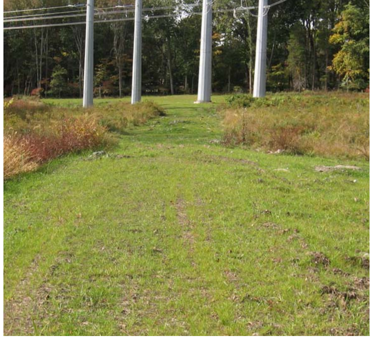
Rimmon Rd/B'Nai: Good vegetative cover has been noted within the restored access road and crane pad areas. Final stabilization has been achieved here.
