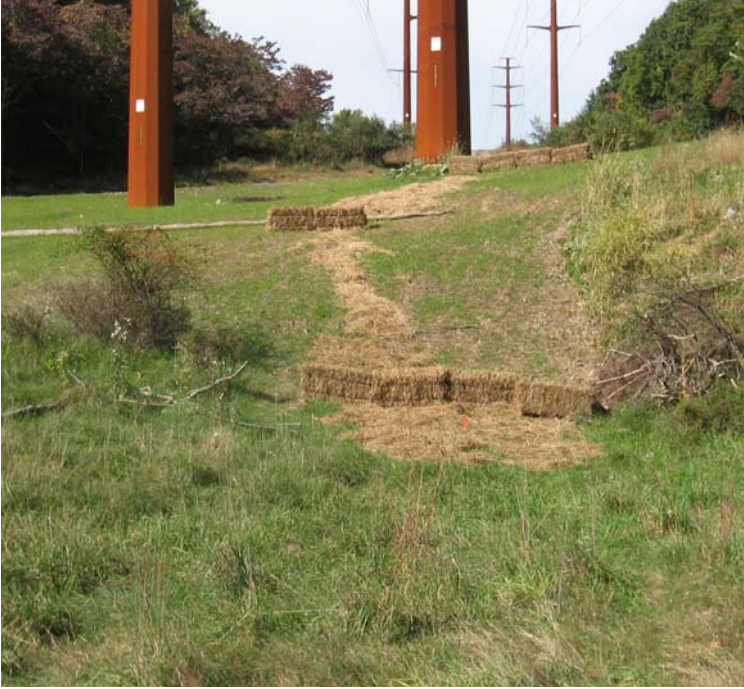
Dogburn Rd south (Orange): The erosive gully near structure #24077 has been graded and temporarily stabilized with mulch.
