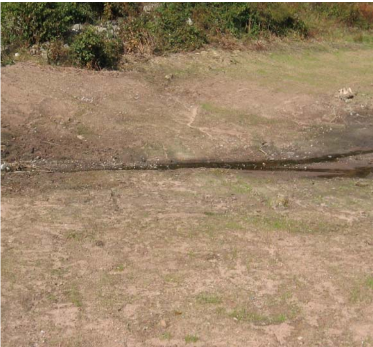
Pease Rd/JCC (Woodbridge): Haybale controls are needed along the intermittent stream within the restored access road.
