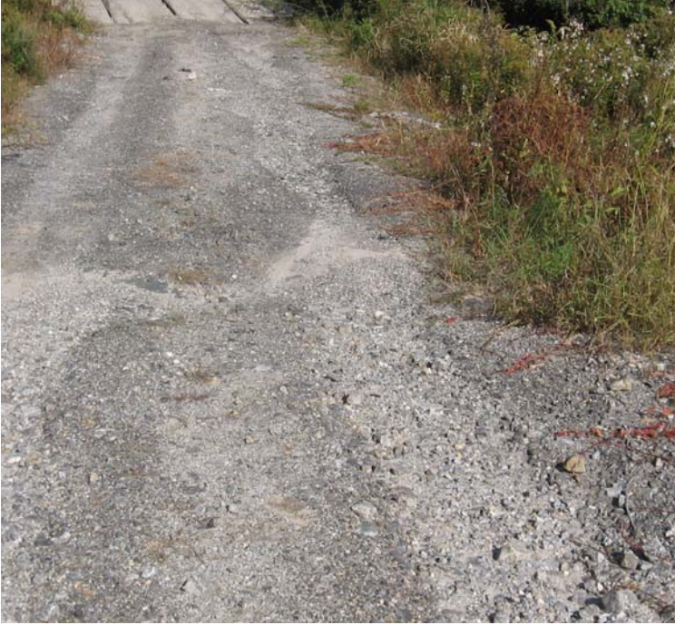
Litchfield Tpk (Bethany): Access road controls are no longer functional near the permanent timber mat crossings.
