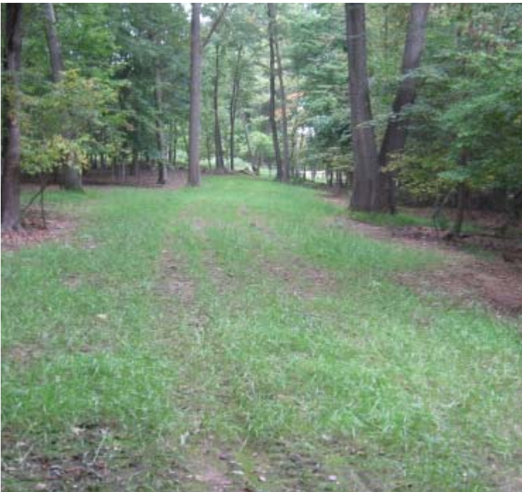
Clearview Ln: A view of the access road restoration efforts near structures #3904/24091. Vegetation growth continues here.
