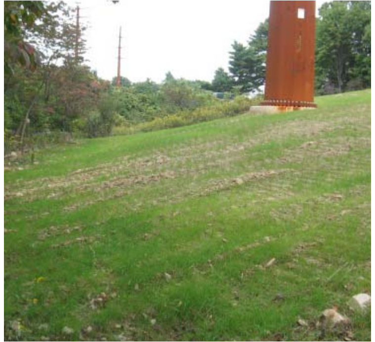
Rt 34: An additional view of vegetative cover near structures #3887/24074. Soils appear stable along the slope at this time.
