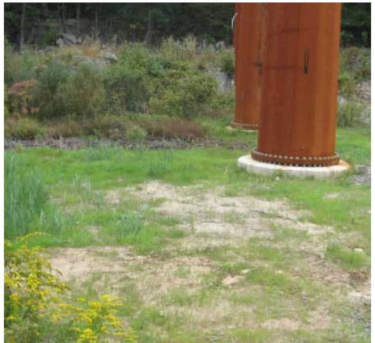
Rt 34: An additional view of the area near structures #3885/24072. Vegetative growth continues to increase here.
