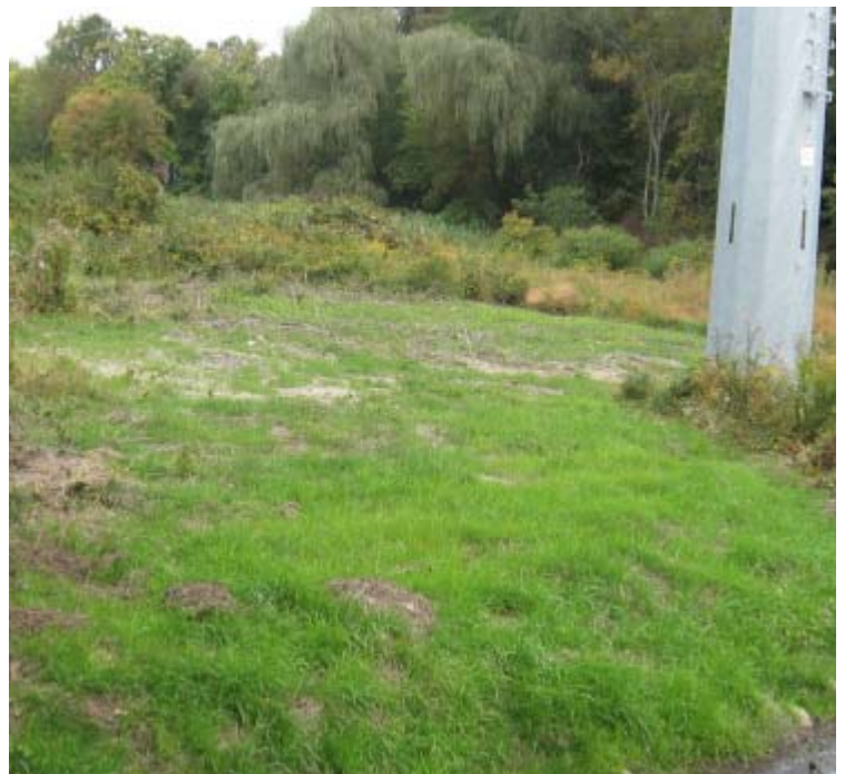
Ansonia Rd (Woodbridge): A view of the restoration efforts near structures # 3914/24101. Approximately 60-65% vegetative cover exists here.
